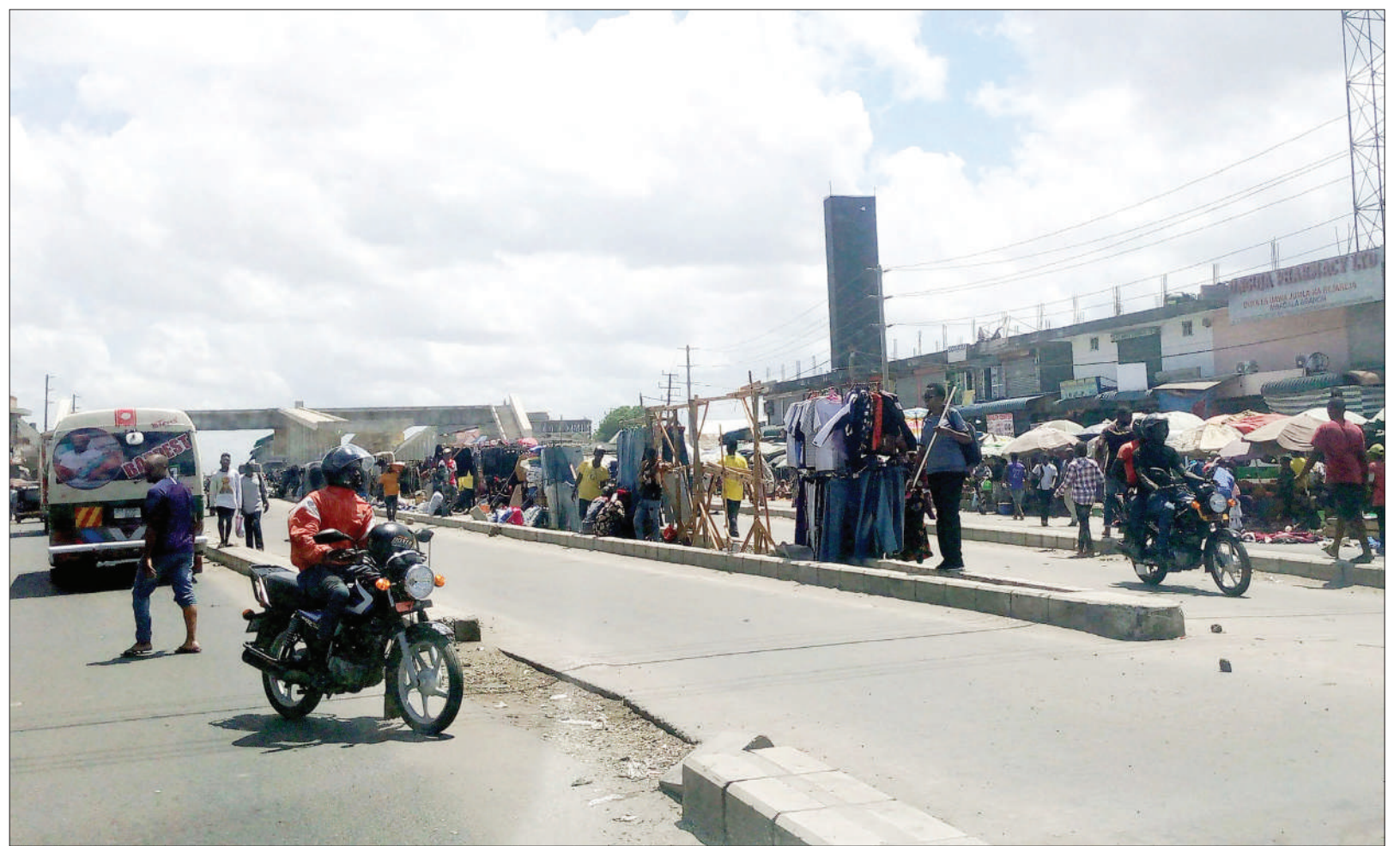
Small traders conduct business just next to the site of the ongoing construction of rapid transit bus infrastructure at a Mbagala Rangi Tatu section of Kilwa Road in Temeke municipality, Dar es Salaam, yesterday. Photo: Correspondent Sabato Kasika
