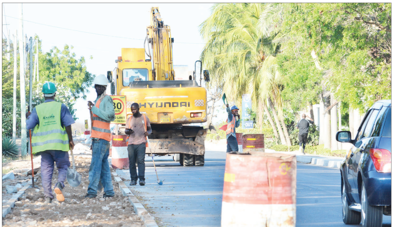
Construction of a pedestrian path in progress yesterday on the side a section of Dar es Salaam's Toure Drive near the Police Officers Mess yesterday. Photo: Correspondent Miraji Msala
