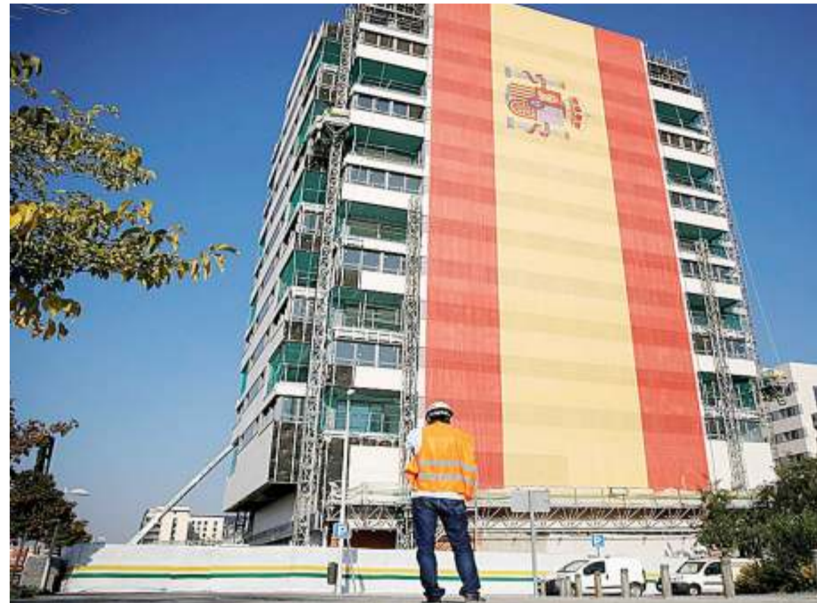
A construction worker looks at a new apartment block draped in a giant Spanish flag in a suburb of Madrid.
