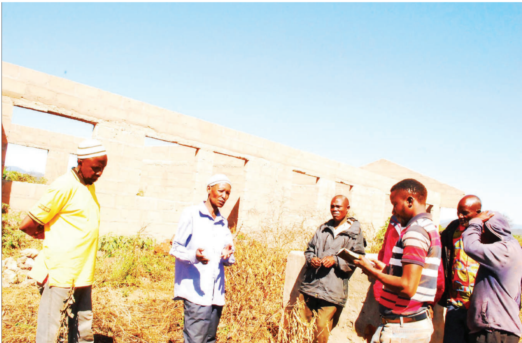
Residents of Ngwandi village in Chamwino District briefs journalists yesterday on a school building they were constructing on self-help basis but which they have abandoned for four years, reportedly for lack of money. They said their children are forced to walk a total of eight kilometers everyday to the nearest school and back. Photo: Correspondent Peter Mkwavila
