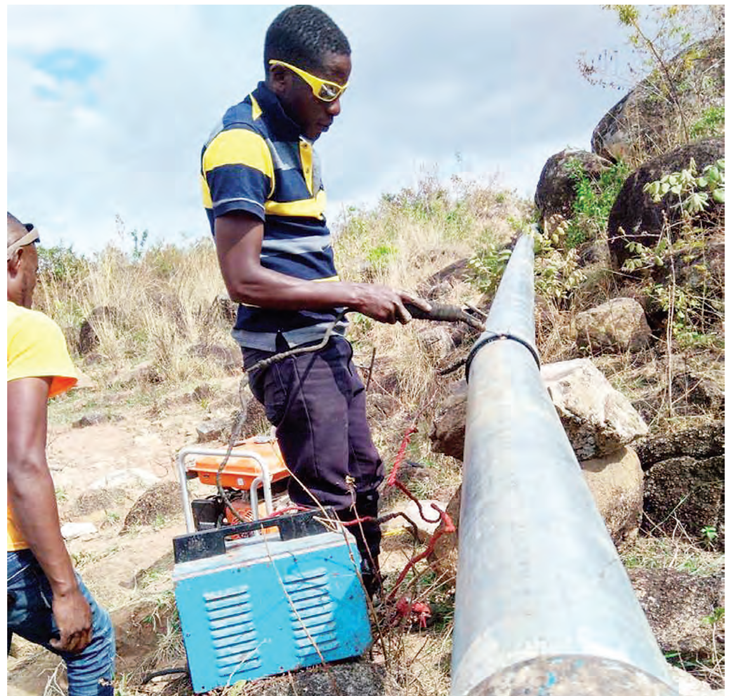
A technician with the Rural Water and Sanitation Agency in Musoma District pictured yesterday working on a major pipe meant to supply water from Lake Victoria to Nyambono and Bugoji wards under an ongoing project being implemented in Musoma Rural constituency. Photo: Guardian Correspondent
