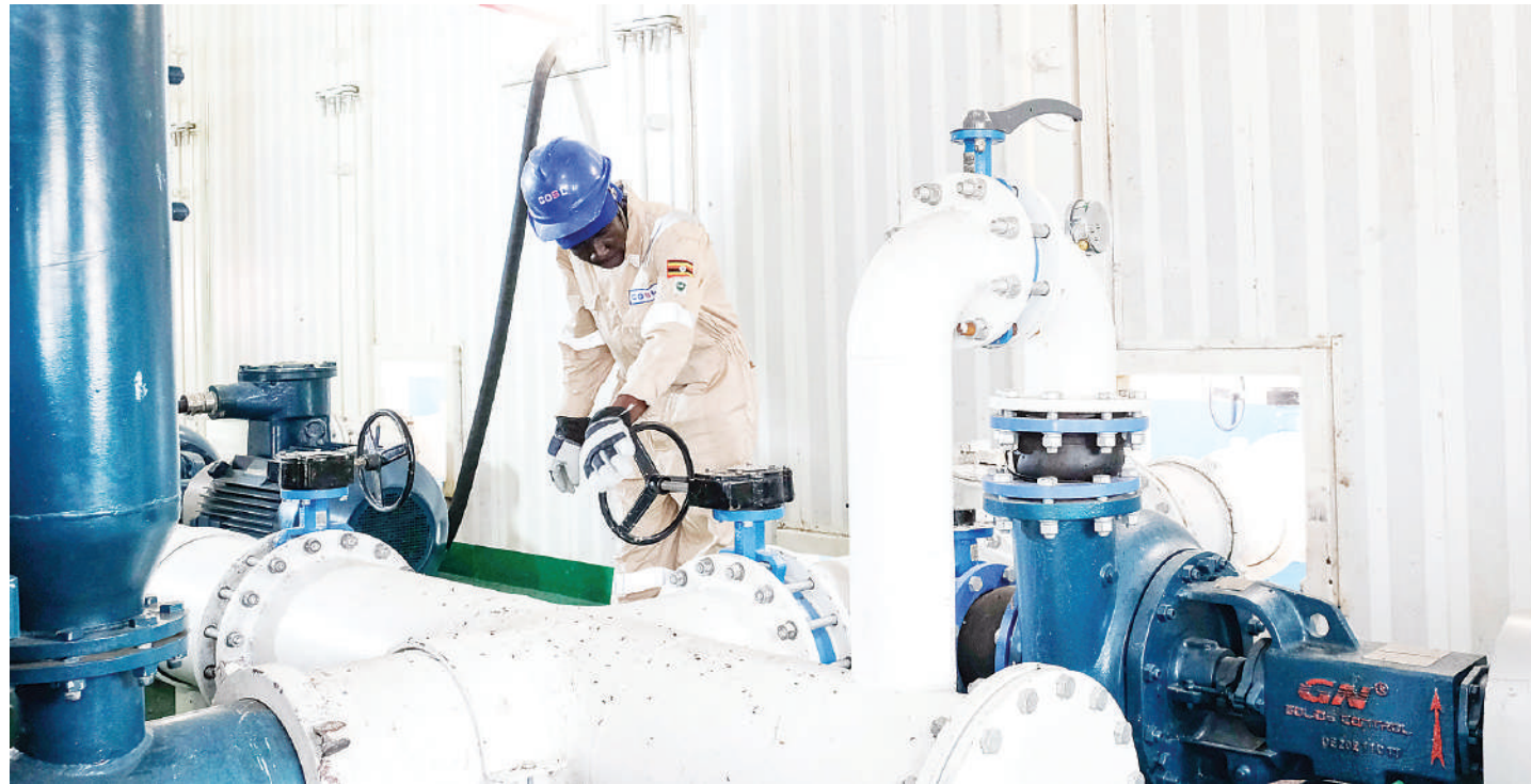
A Ugandan worker operates the mud pump unit at the Kingfisher oil field in Kikuube, Uganda, Jan. 24, 2023. Xinhua
