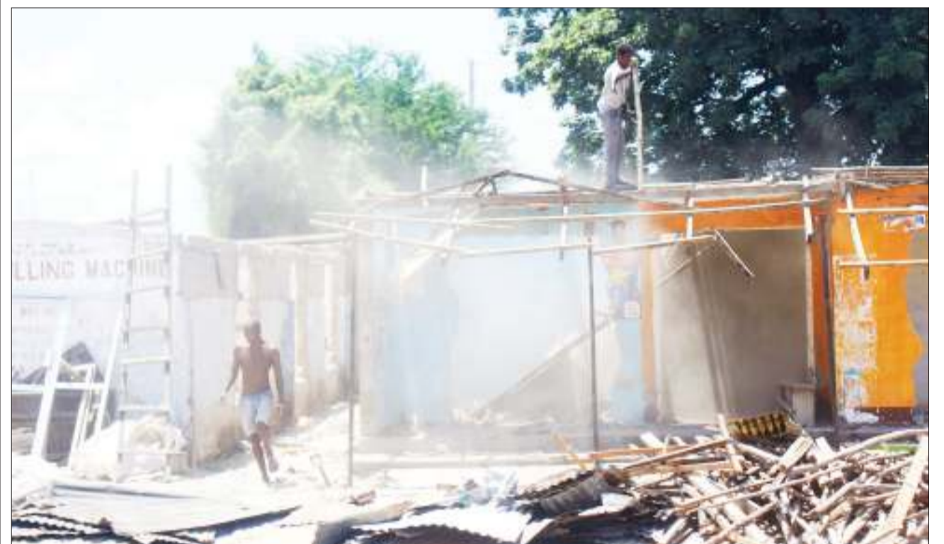
Residents of Dar es Salaam's Ukonga suburb pull down their houses and other structures yesterday to pave the way for the implementation of the Standard Gauge Railway project. Photo: Halima Kambi
