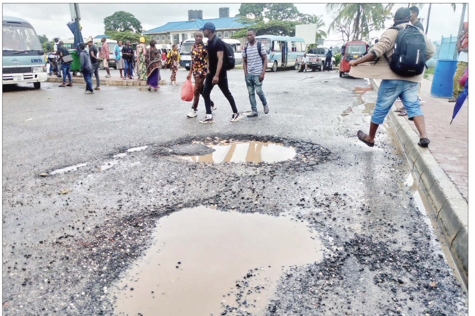
Road traversing the Mbezi Mwisho commuter bus stand in Dar es Salaam's Ubungo municipality badly damaged, as witnessed by our Roving Correspondent yesterday.
