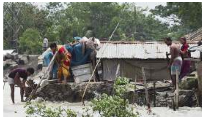
People fix their damaged homes amid high waters in Khulna as Cyclone Fani lashes Bangladesh. AFP
