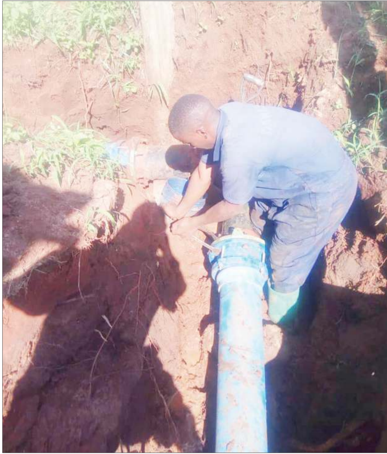
Dar es Salaam Water and Sanitation Authority technician Oscar Godwin tightens a water pipe in the city's Luguruni suburb yesterday in a bid to stop leakage. Photo: Guardian Photographer
