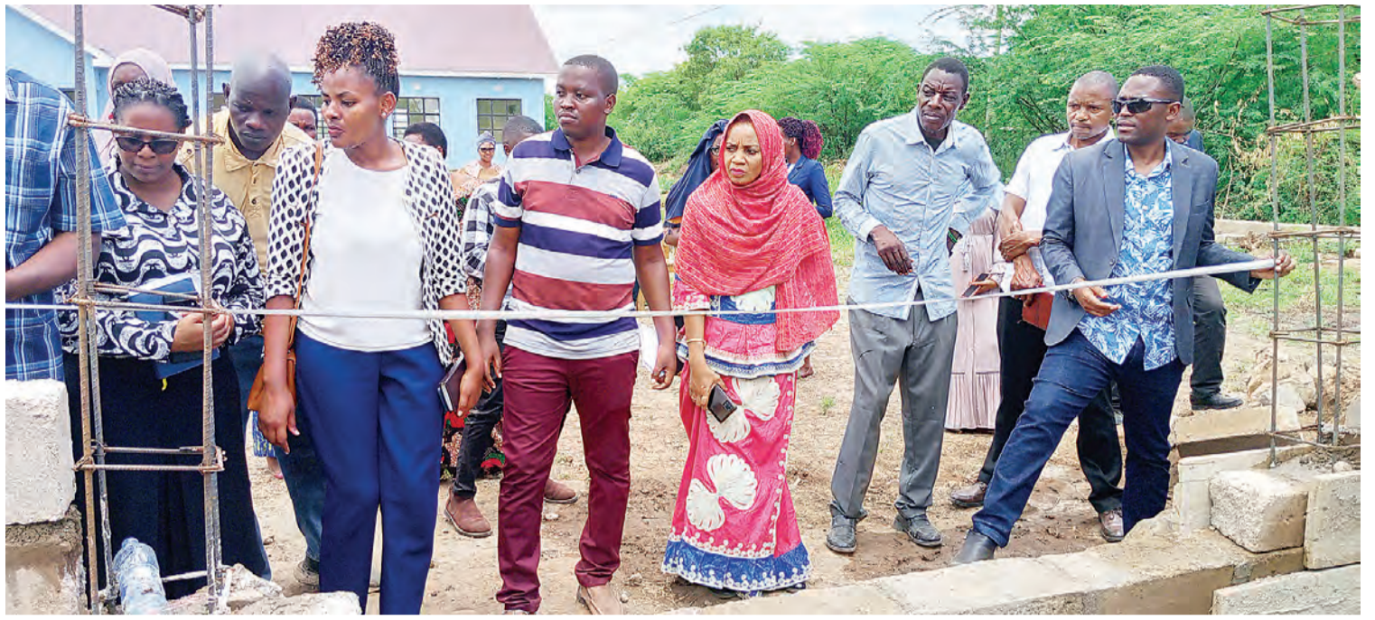
Simanjiro district commissioner Dr Suleiman Serera (R) pictured during a tour on Thursday taking measurements of the proposed gate to the concrete fence being built mainly with a view to enhancing security around Mirerani ward's Songambebe Primary School dormitory for children with special needs. Photo: Correspondent Gift Thadey
