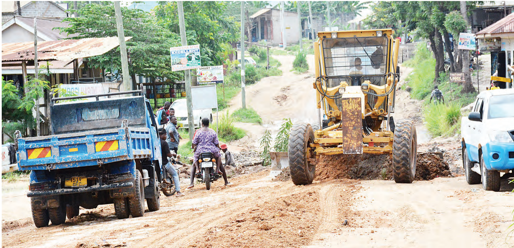
Construction of a storm drain gets well under way beside a newly built road in Mbulu District, Manyara Region, as found earlier this week. Photo: Correspondent Jumanne Juma
