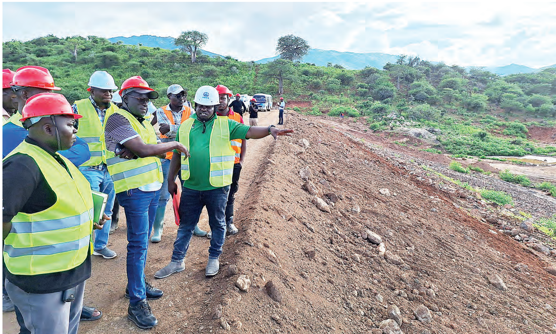
National Irrigation Commission dam construction project engineer Salehe Ramadhani (3rd-L) shows visiting media editors a 12-billion-litre dam under construction at Membe in Chamwino District, Dodoma Region, yesterday. Photo: Correspondent Joseph Mwendapole
