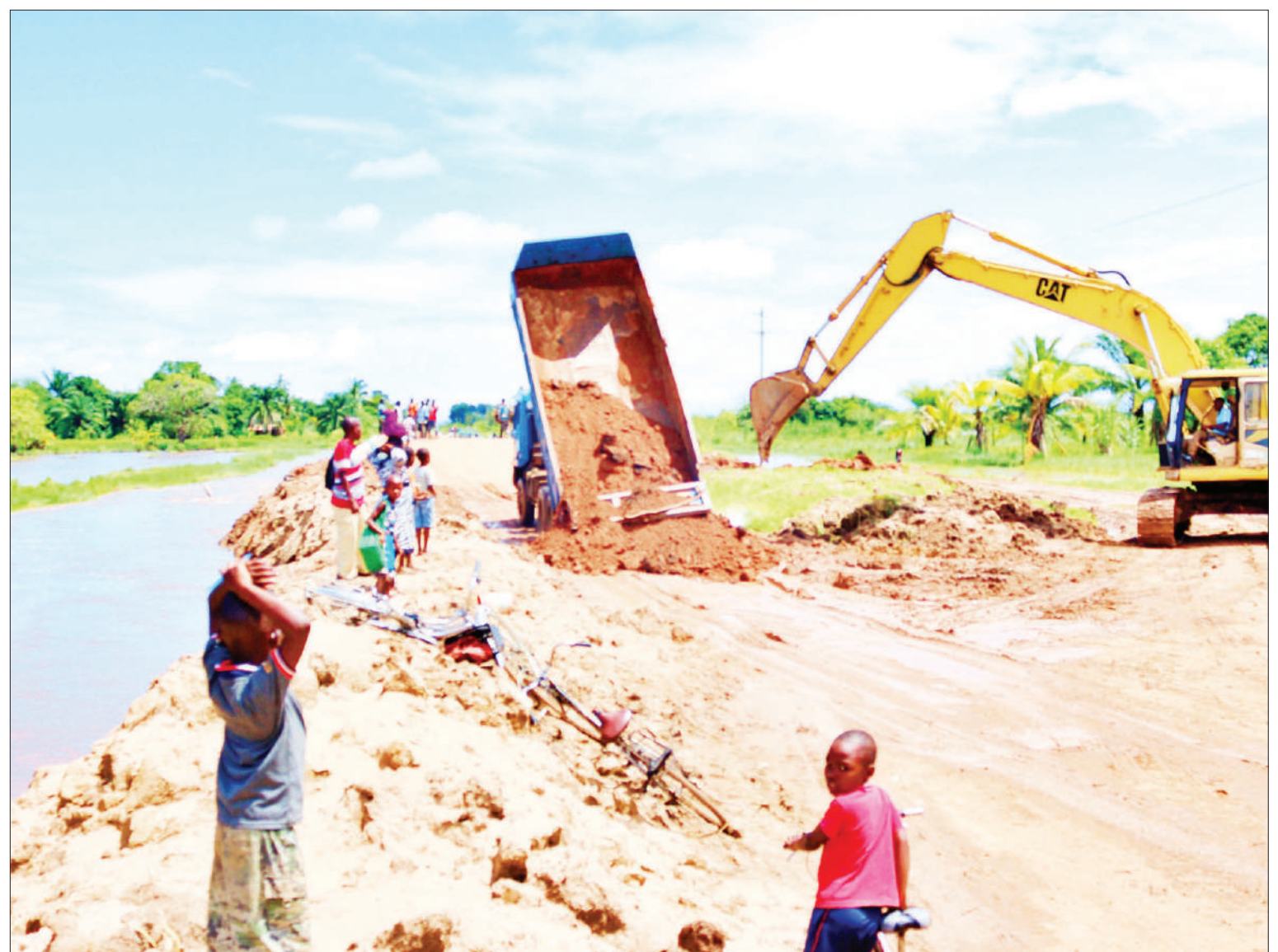
Road construction in progress at Misegese village in Malinyi, Morogoro Region, last week following damage due to the flooding of the nearby River Furua. Photo: Guardian Correspondent
