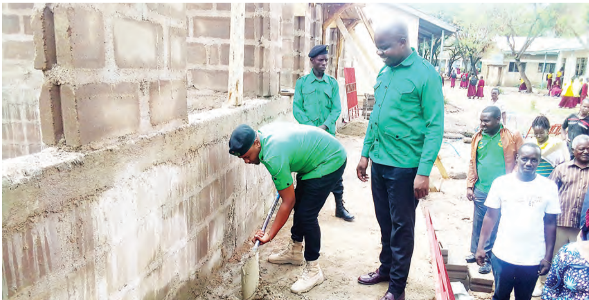
Baraka Shemahonge (L), the CCM youth wing's Shinyanga regional chairman, participates in the construction of classrooms at Uhuru Secondary School in Shinyanga municipality yesterday. Behind him is the wing's Shinyanga Urban district chairman, Dotto Joshua. Photo: Correspondent Marco Maduhu
