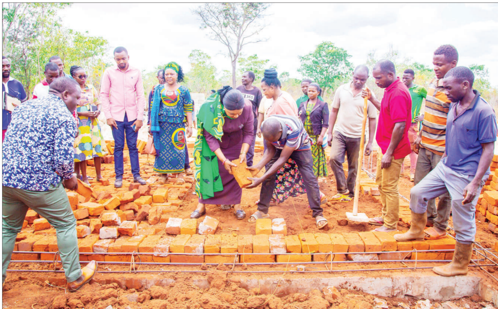
Jenista Mhagama (C, in purple dress), Minister of State in the Prime Minister's Office (Policy, Parliament and Coordination), joins self-help efforts in construction work at Lugagara Secondary School at Kilagano in Songea Rural District yesterday. Photo: PMO
