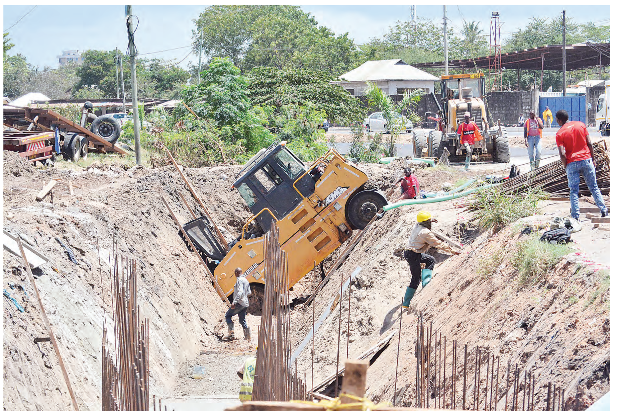
GRADER IN TROUBLE: A grader deployed to help in rehabilitating Dar es Salaam's Shekilango Road unable to do the work it was supposed to do, having tumbled into sewage trench. Correspondent Miraji Msala captured the scene yesterday.
