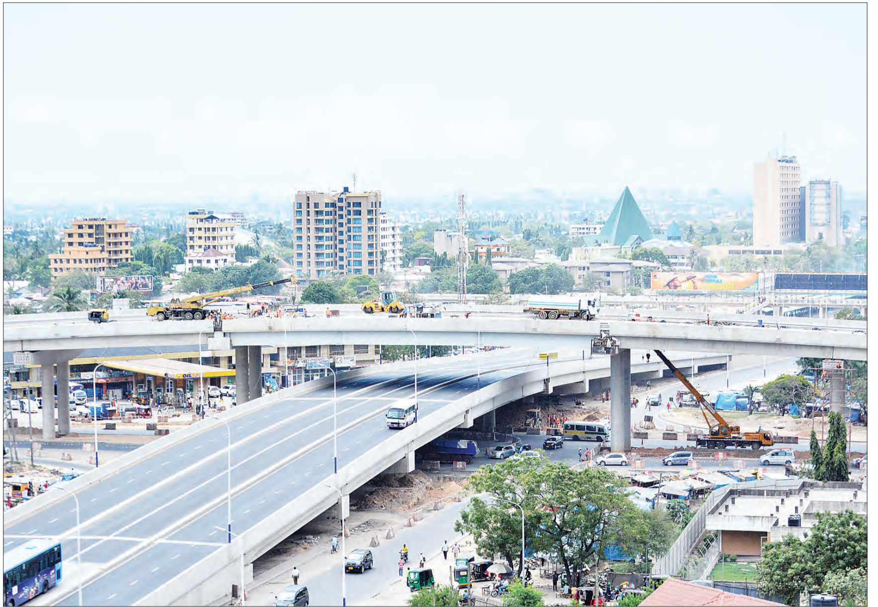
Completion of work on Dar es Salaam's Ubungu interchange well in sight, with contractors putting what they call finishing touches to the ultramodern facility - as found yesterday. Photo: Correspondent Miraji Msala
