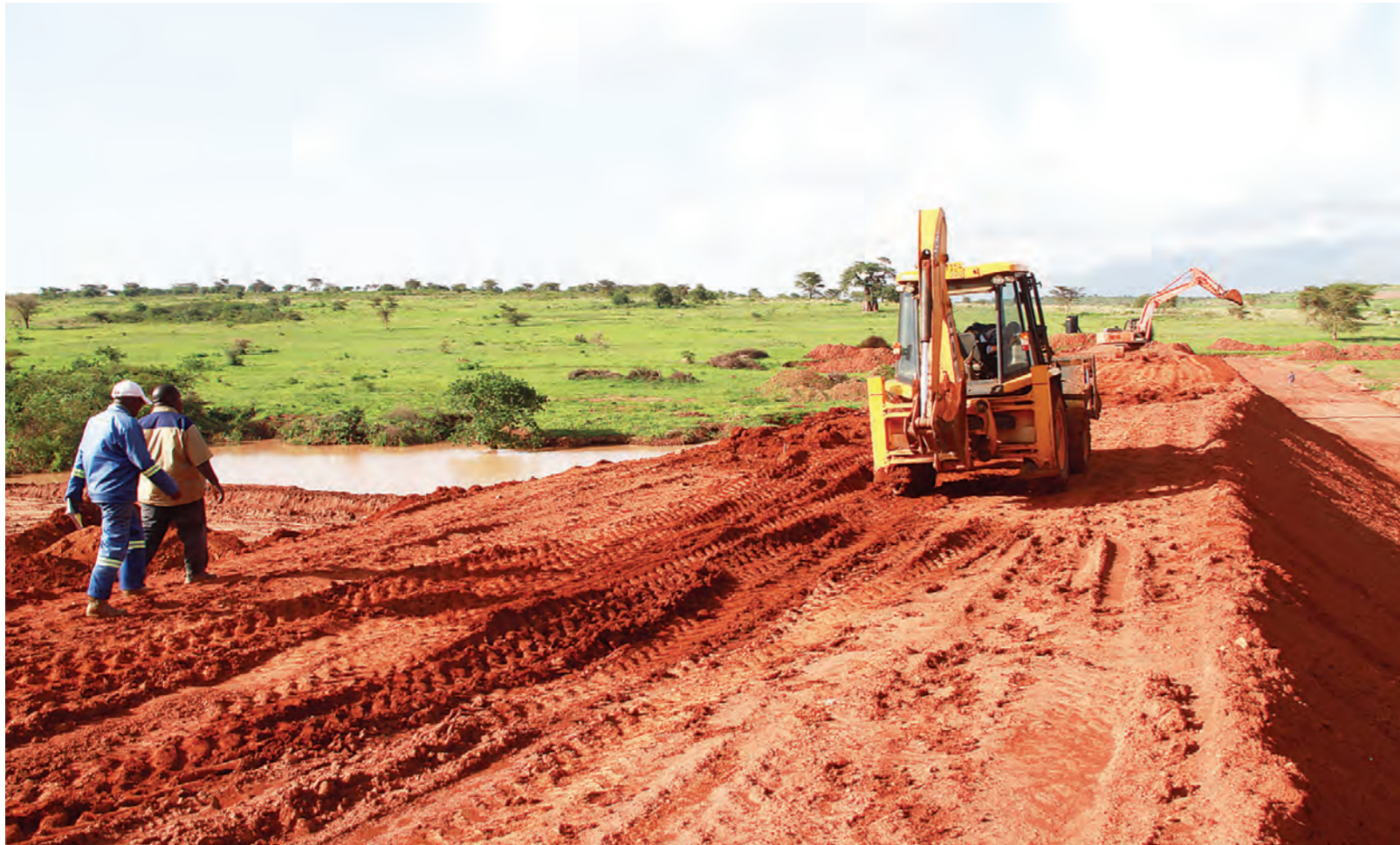
Construction of irrigation infrastructure under way at a Farm for the Future farm in Kilolo District, Iringa Region, at the weekend. The firm is a Southern Agricultural Growth Corridor of Tanzania (SAGCOT) stakeholder. Photo: Guardian Correspondent
