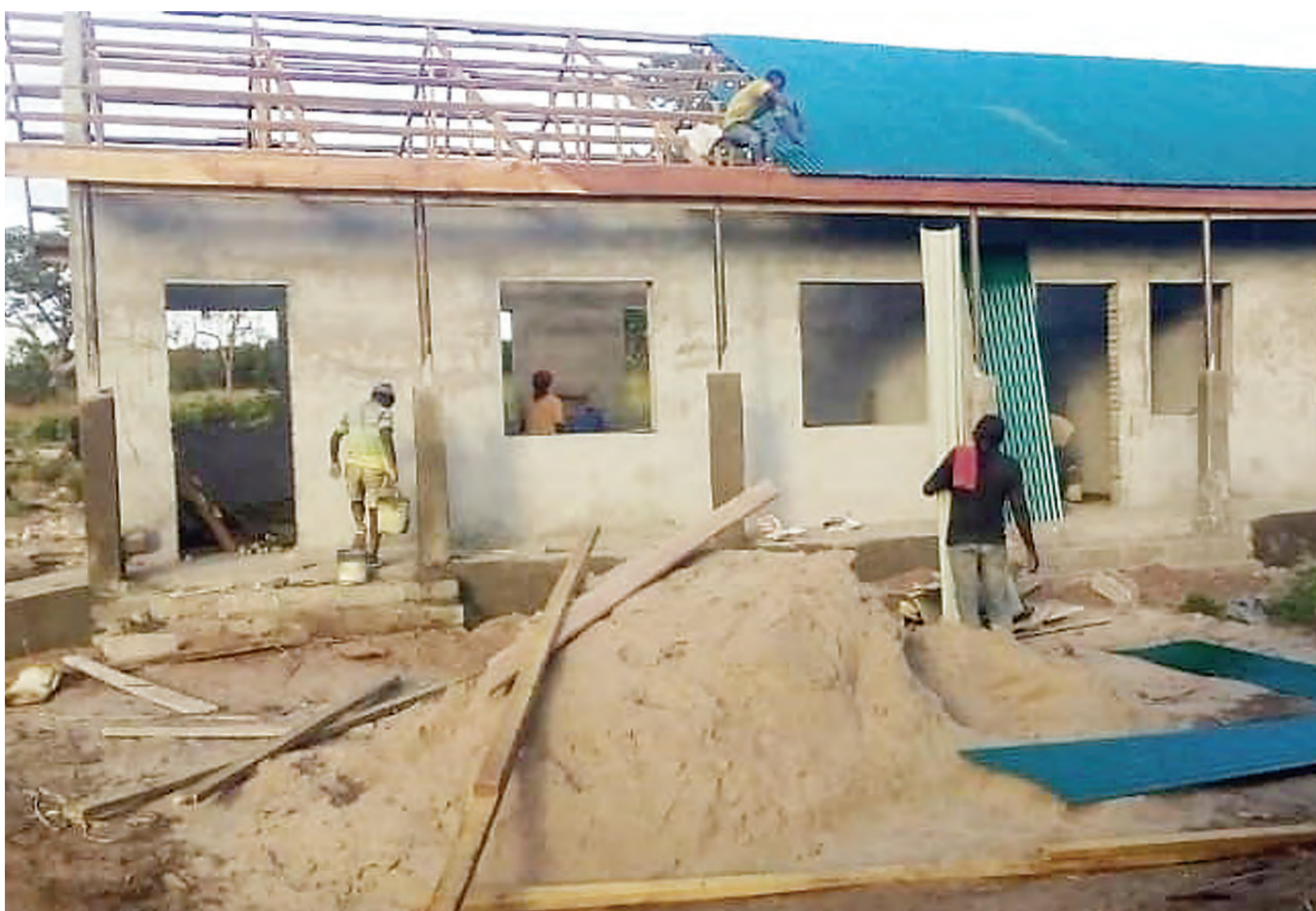
Technicians at work during the construction of one of the classrooms of Mangirikiti secondary school in Liwale district, Lindi region earlier this week which is expected to reduce the shortage of classrooms at the school. Photo: Guardian correspondent
