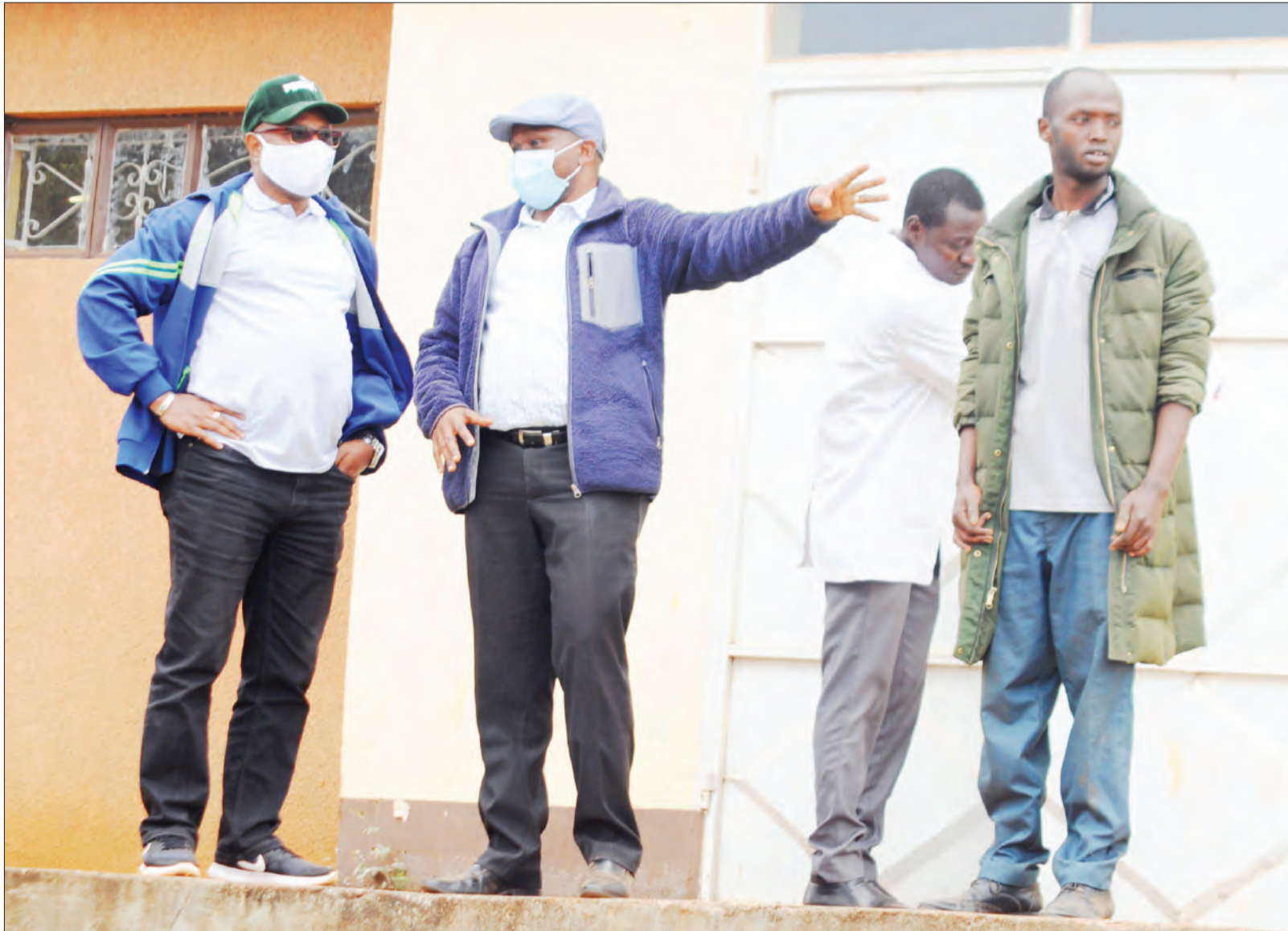
Karatu district commissioner Abbas Kayanda (L) is briefed yesterday on the ongoing construction of a mortuary at Oldean health centre in Arusha Region. Photo: Correspondent Woinde Shizza
