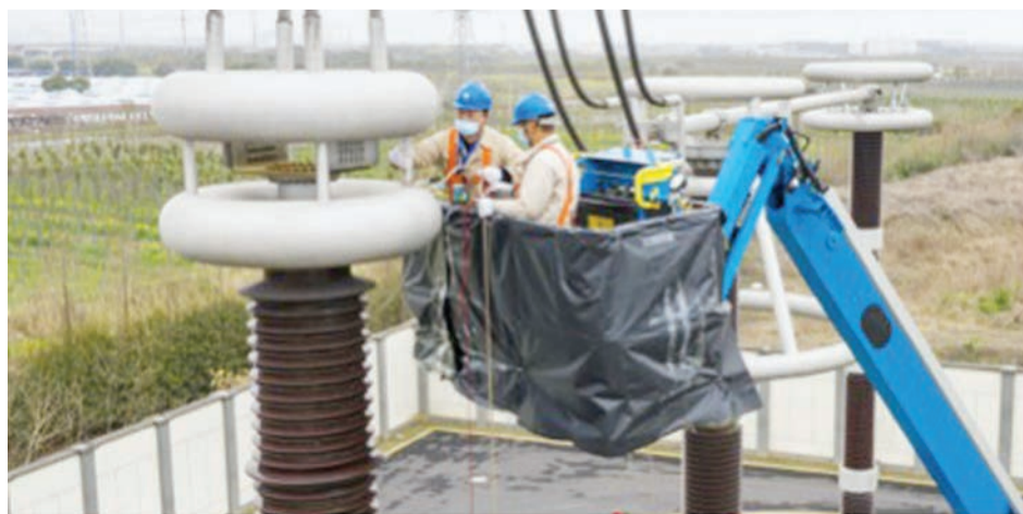
Devices and cables at a 1,000-KV ultrahigh voltage transformer substation in Suzhou, east China's Jiangsu province are overhauled by technicians from the power transmission and distribution company under the State Grid Jiangsu Electric Power Co., Ltd., March 13, 2021. (File photo)
