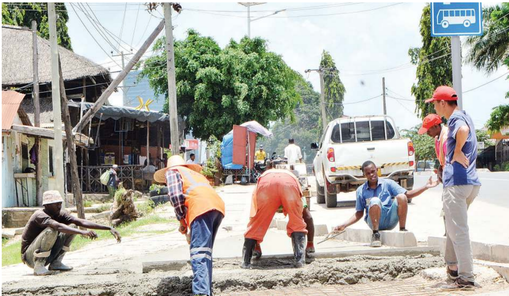
China Civil Engineering Construction Corporation workers lay the groundwork for the installation of a commuter bus stop earlier this week as part of the ongoing construction of the road linking Dar es Salaam's Sinza Kijiweni and Tandale suburbs. Photo: Correspondent Miraji Msala
