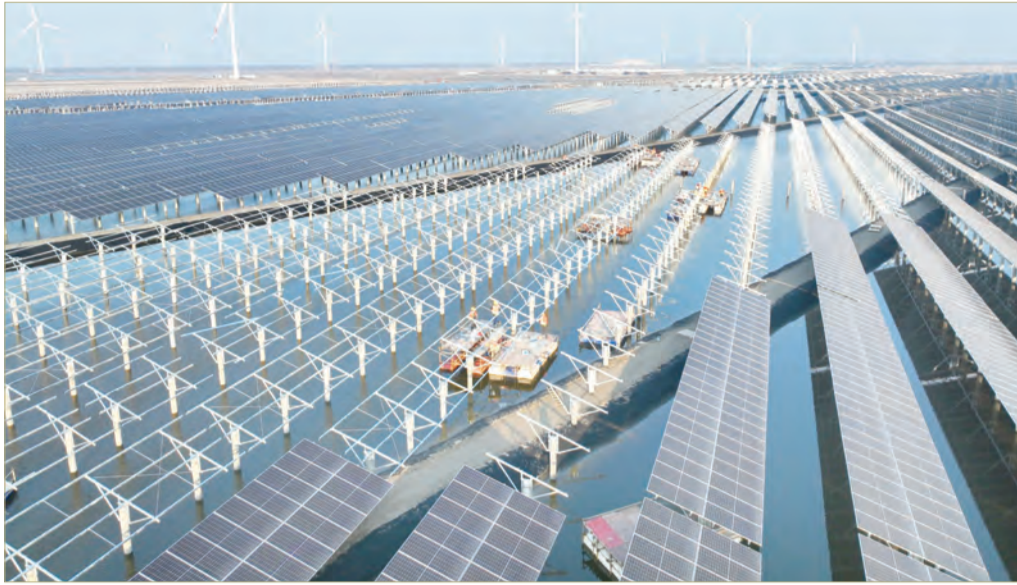
Photovoltaic panels are installed in a fish farm in Rudong county, Nantong, east China's Jiangsu province, Feb. 20, 2023. (Photo by Xu Congjun/People's Daily Online)
