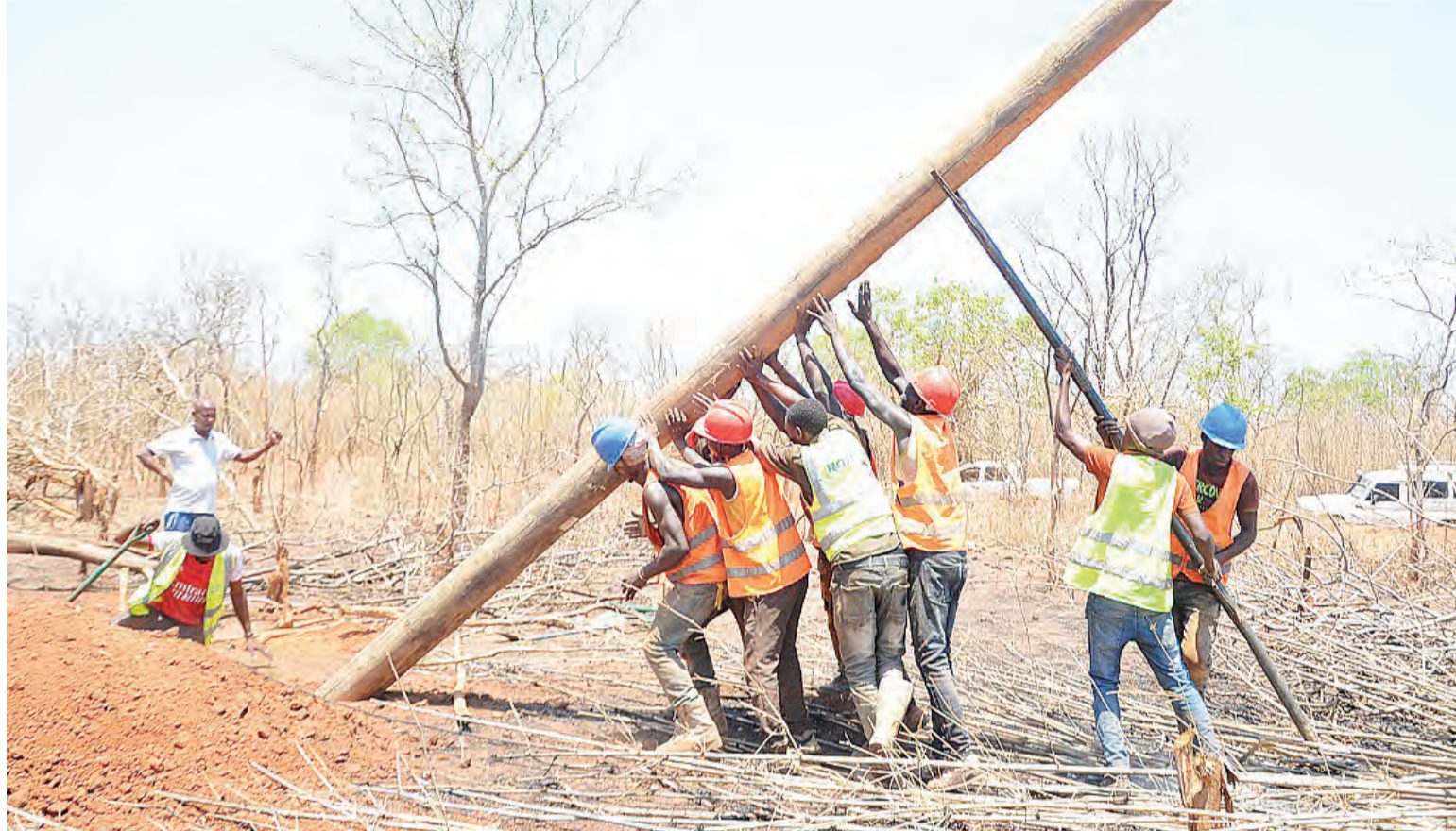
Technicians erect electric pole in one of the villages in Nanyumbu District, Mtwara Region recently. Photo courtesy of REA
