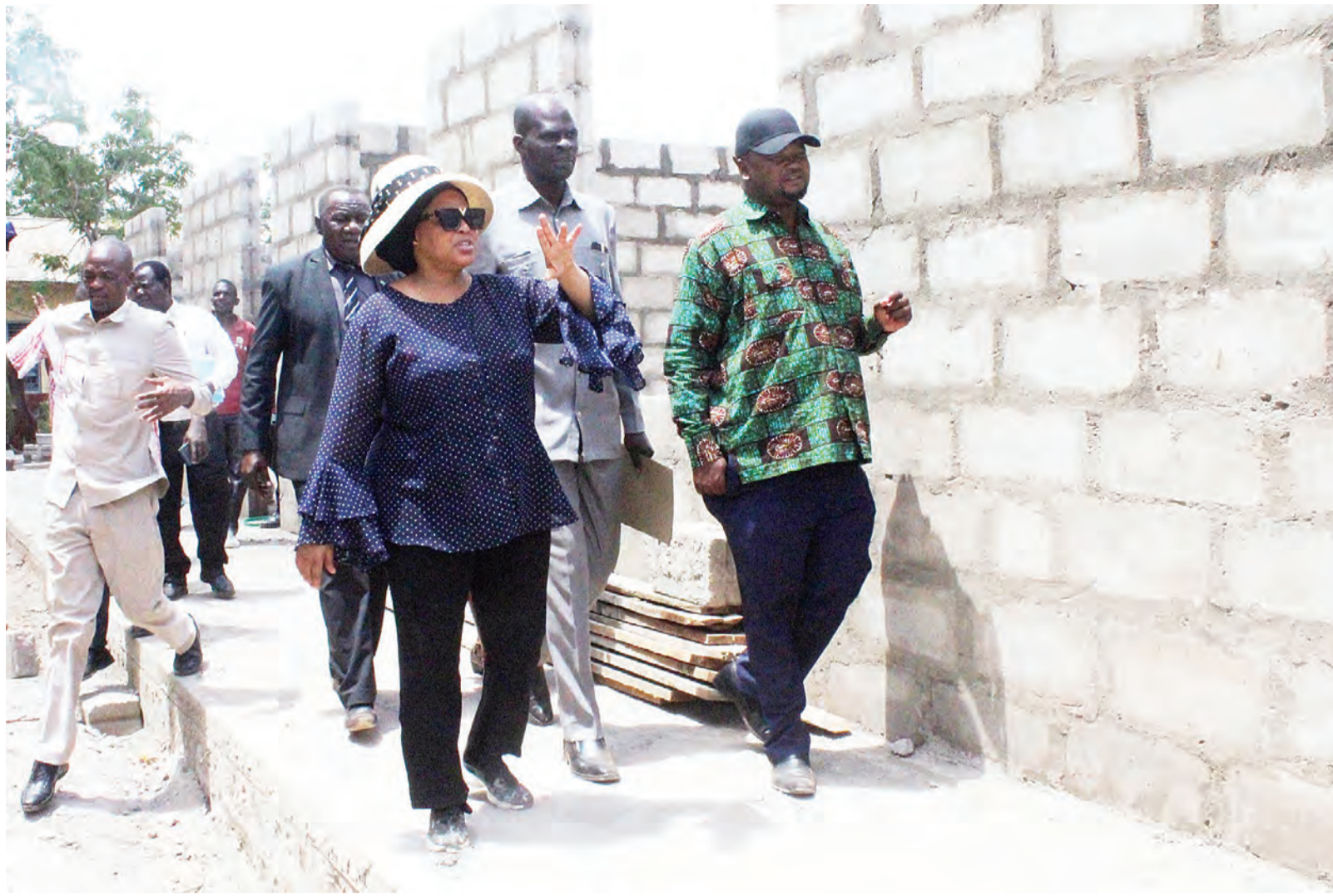
Shinyanga regional commissioner Sophia Mjema (in hat) has an eyewitness account of the ongoing construction of classrooms at Mwalimu Nyerere Secondary School at Segese in Msalala Council, Kahama District, earlier this week. Right is Kahama district commissioner Festo Kiswaga. Photo: Correspondent Marco Maduhu
