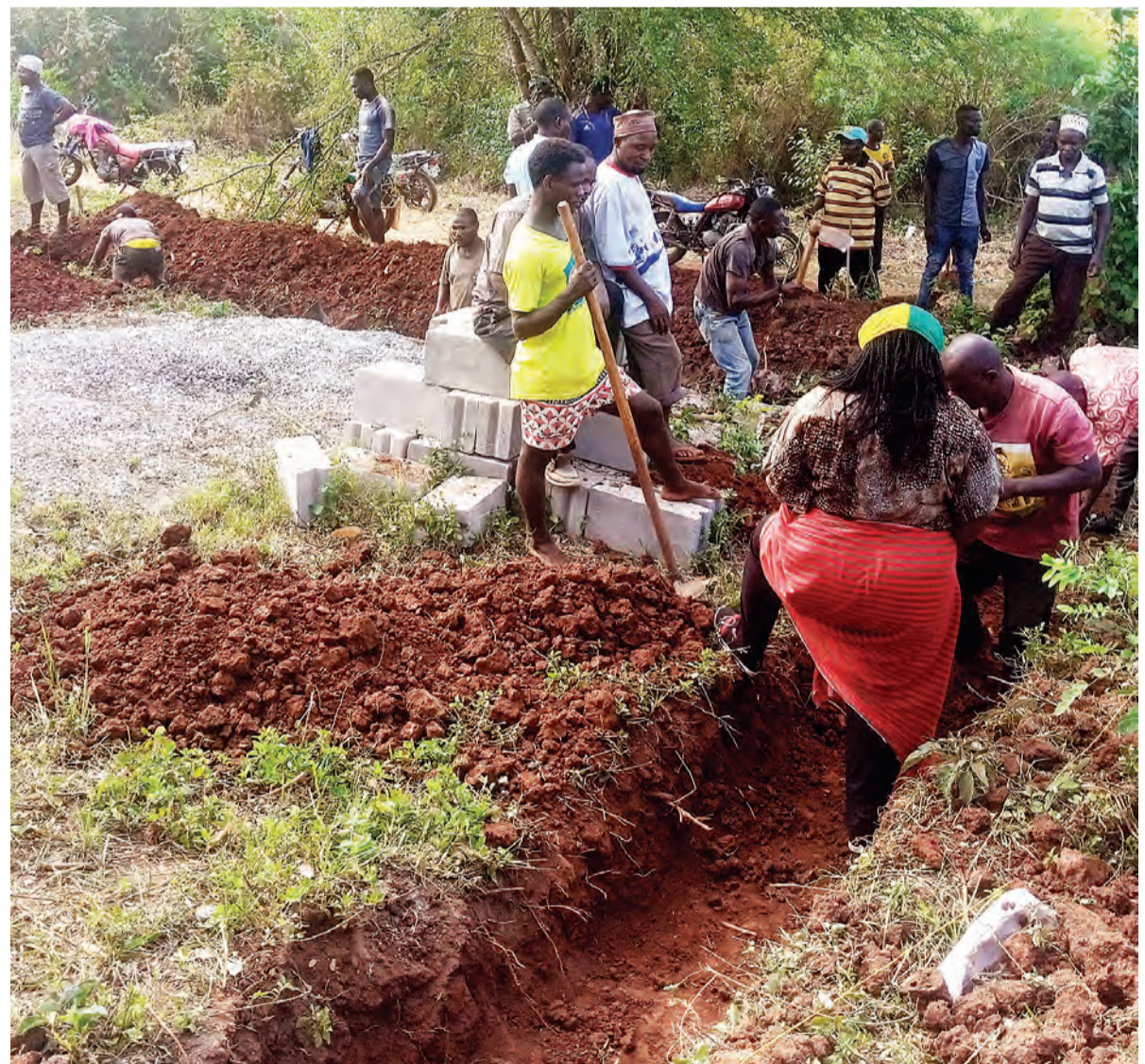
Residents of Songa in Muheza District, Tanga Region, take part in the preliminary stages of the construction of four secondary school classrooms on Thursday. Photo: Correspondent Steven William
