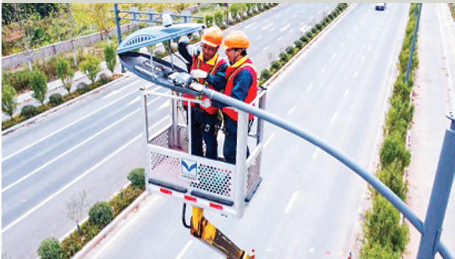
Technicians install a smart street lamp in Jinyi New Area, Jinhua, east China's Zhejiang province, Oct. 11, 2022. (Photo by Chen Jun/People's Daily Online)
