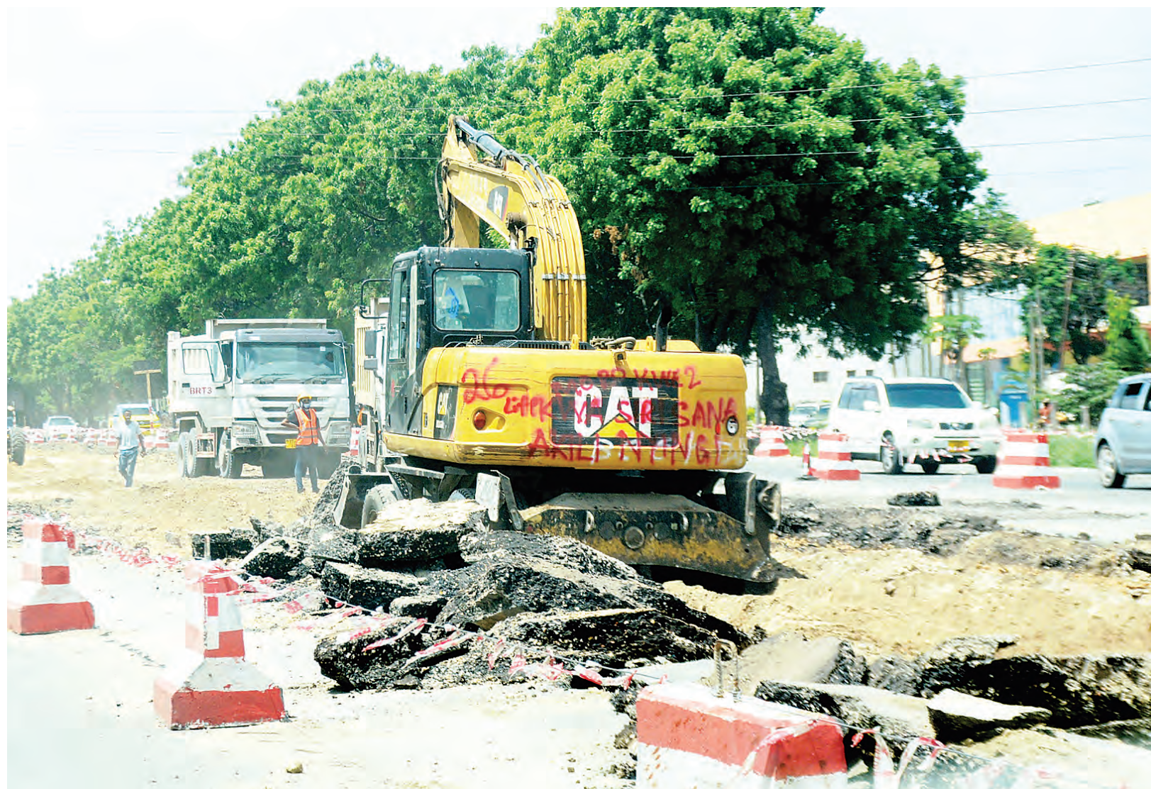
Preparations for the implementation of the third phase of Dar es Salam's rapid bus transport project along the Gerezani to Gongo la Mboto stretch of Nyerere Road well in progress yesterday at the Sigara (TCC) section. Photo: Correspondent Jumanne Juma
