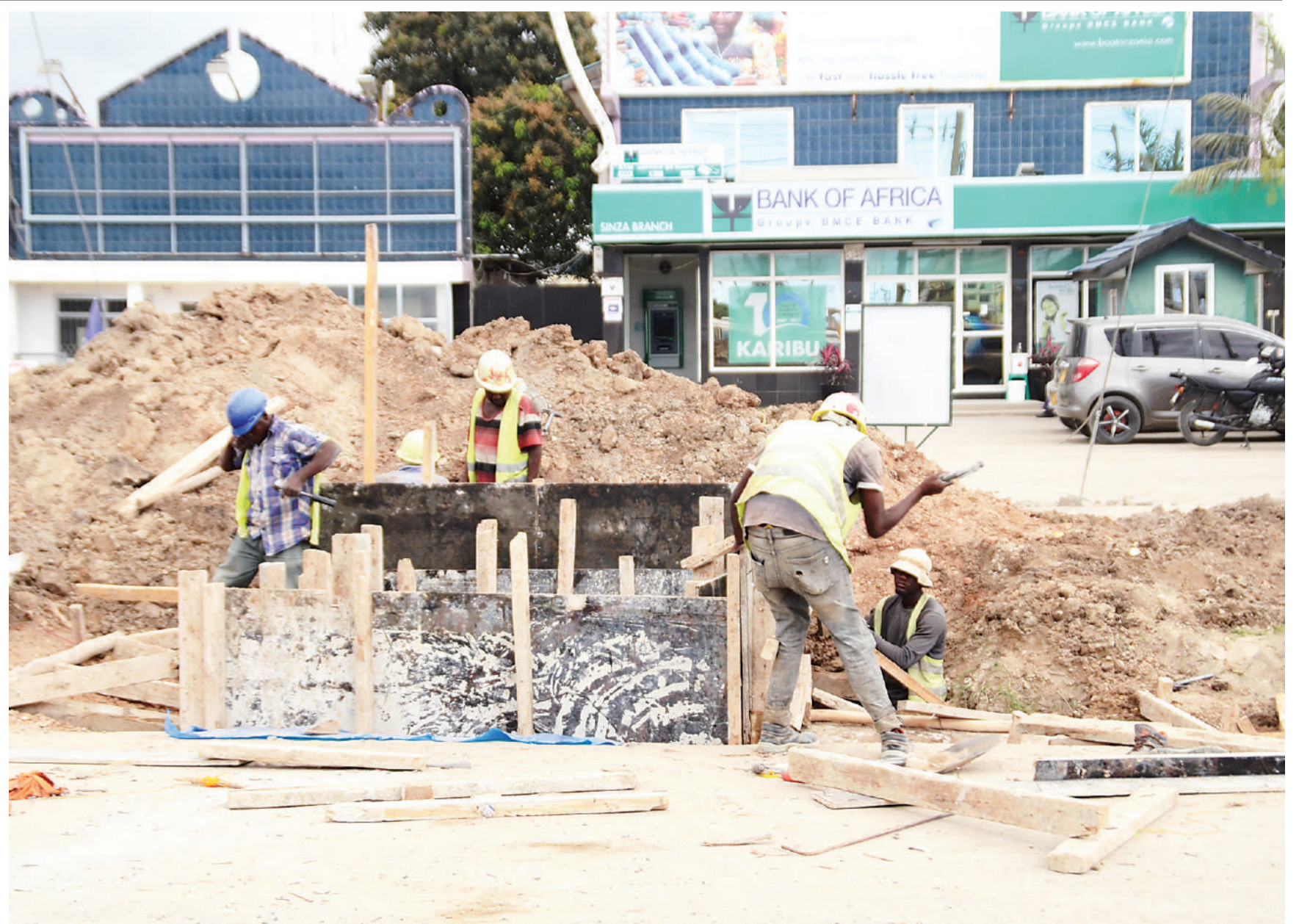
Construction of sewage system chamber under way yesterday as part of the ongoing rehabilitation of Dar es Salaam's Shekilango Road. Photo: Correspondent Jumanne Juma
