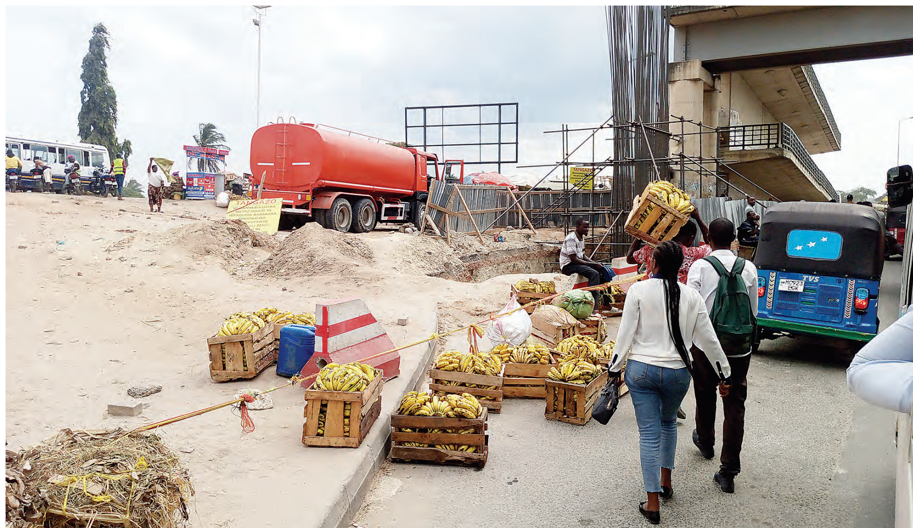
Apparently for lack of an ideal site where to conduct business, fruit vendors move to try it out at this unauthorised roadside in Dar es Salaam's Kimara Mwisho suburb on Saturday. But they were soon ordered out to pave the way for the ongoing rehabilitation and expansion of Morogoro Road. Photo: Correspondent Sabato Kasika
