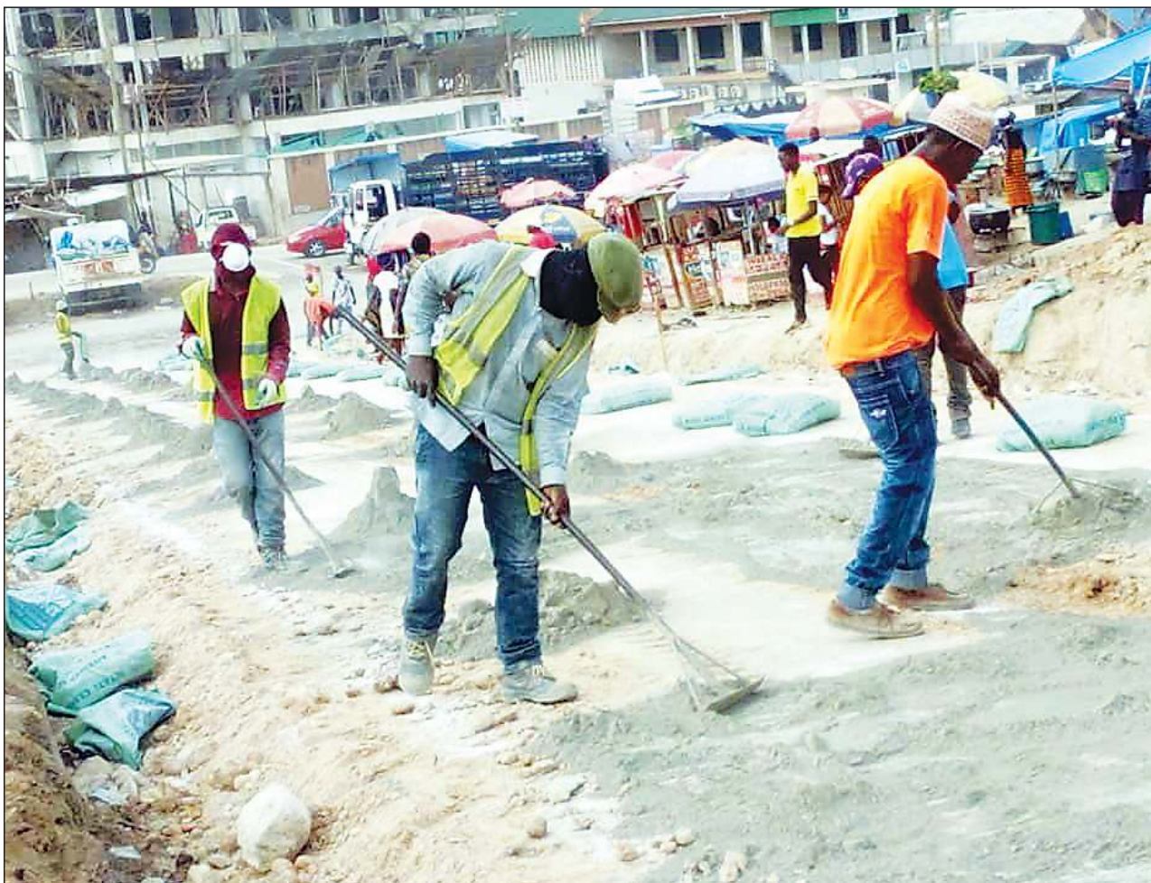
Morogoro road expansion is going on well at Mbezi Mwisho in the outskirts of Dar es Salaam yesterday. Photo: Correspondent Sabato Kasika
