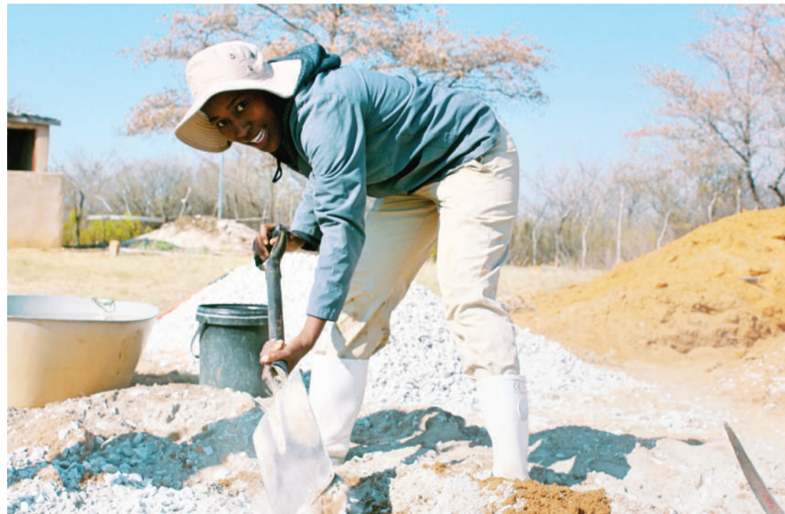
Atamelang Matala mixes concrete to build a biogas digester at Betesankwe Village in the Southern District, Botswana, on Sept. 2, 2022. Xinhua
