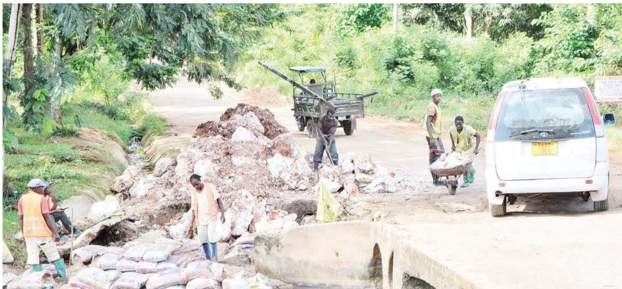
Rehabilitation of Dar es Salaam's Goba-Tegeta 'A' bridge, which has been damaged by weeks of pounding rain, well in progress yesterday. Photo: Correspondent Miraji Msala
