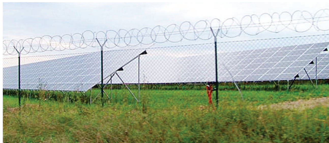
An 8.5MW solar power plant in Rwamagana District.
