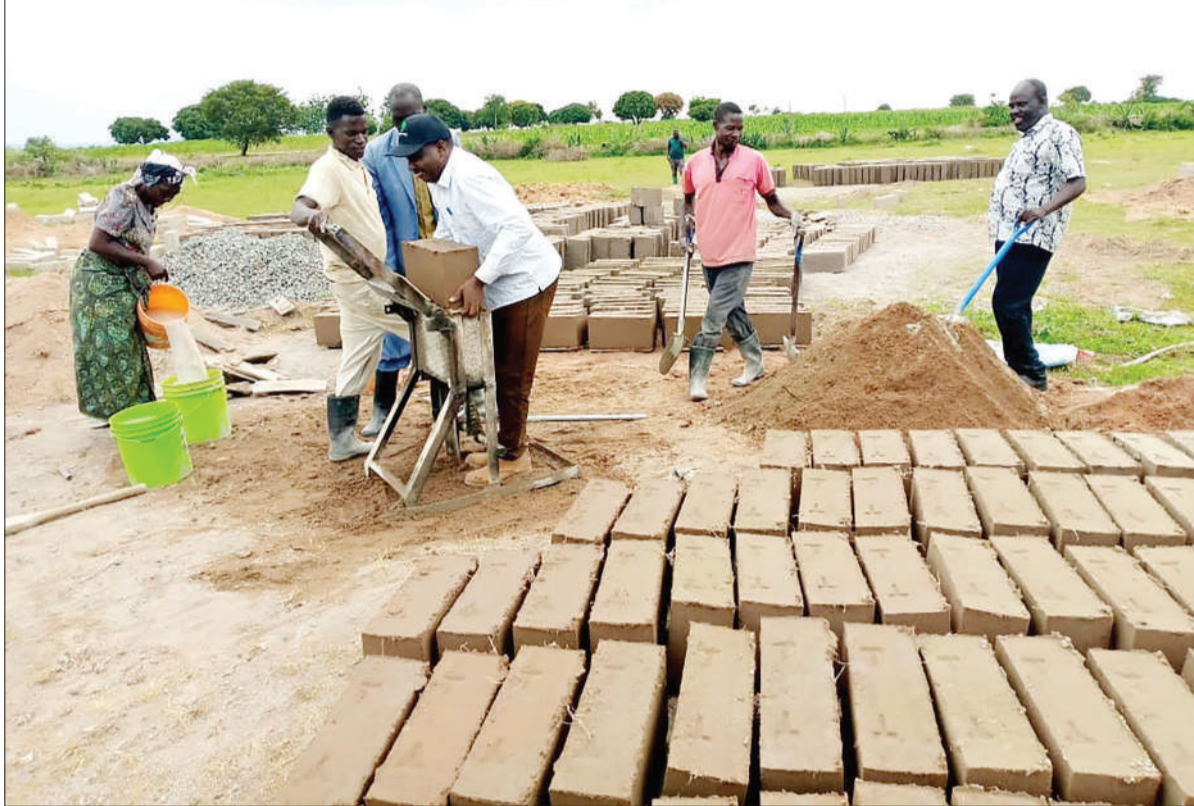
Musoma district commissioner Dr Khalfan Haule (in cap) takes part in the making of bricks for use in construction work at a secondary school at Muhoji village yesterday. Photo: Guardian Correspondent
