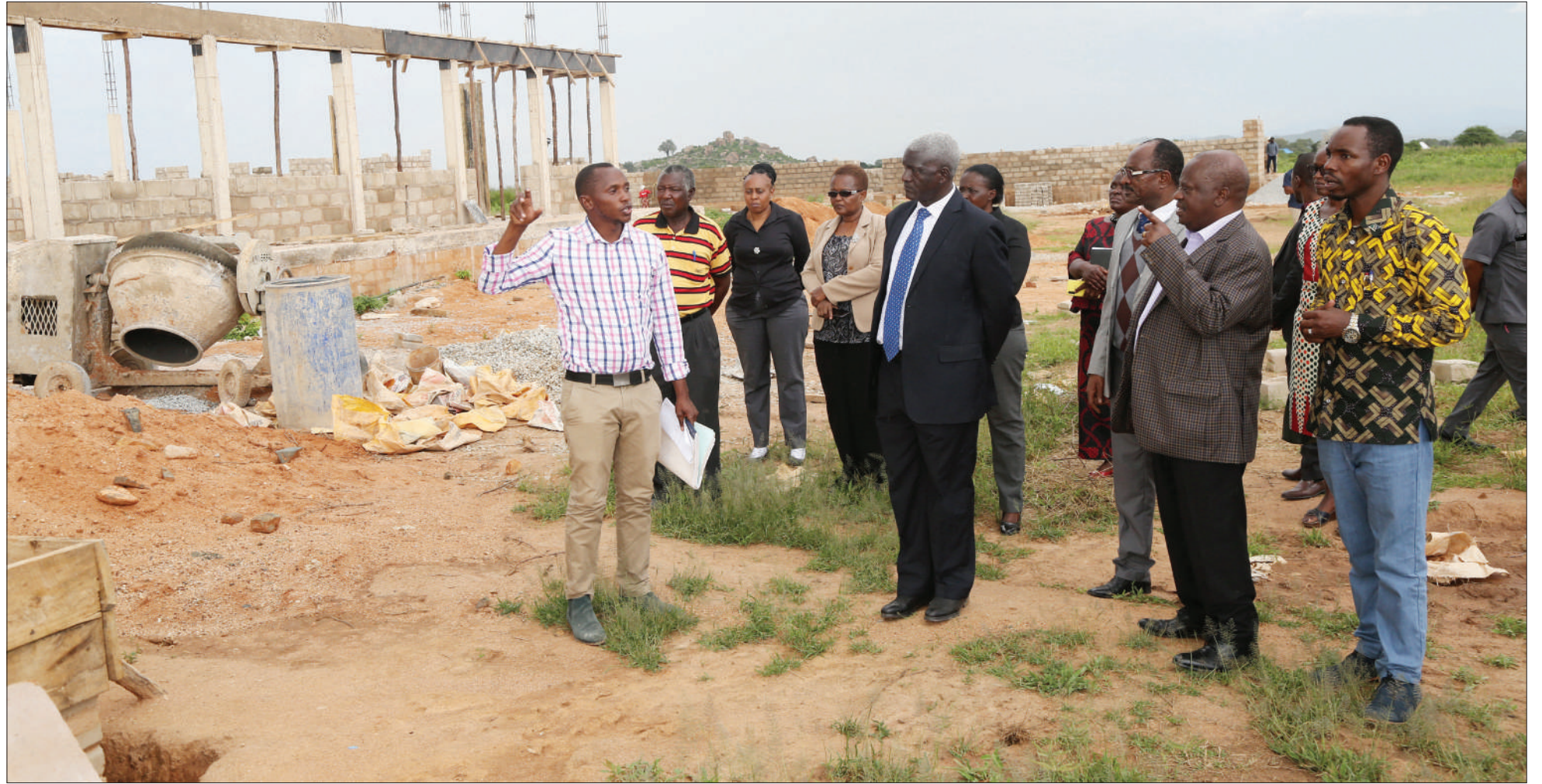
Howard Fuka (L), a consultant coordinating the construction of Bunge Girls High School at Kikombo in Chamwino District, briefs a delegation including National Assembly Speaker Job Ndugai (2nd-R) and Dodoma regional commissioner Dr Binilith Mahenge (C, in suit) on an inspection visit at the construction site yesterday. Photo: National Assembly
