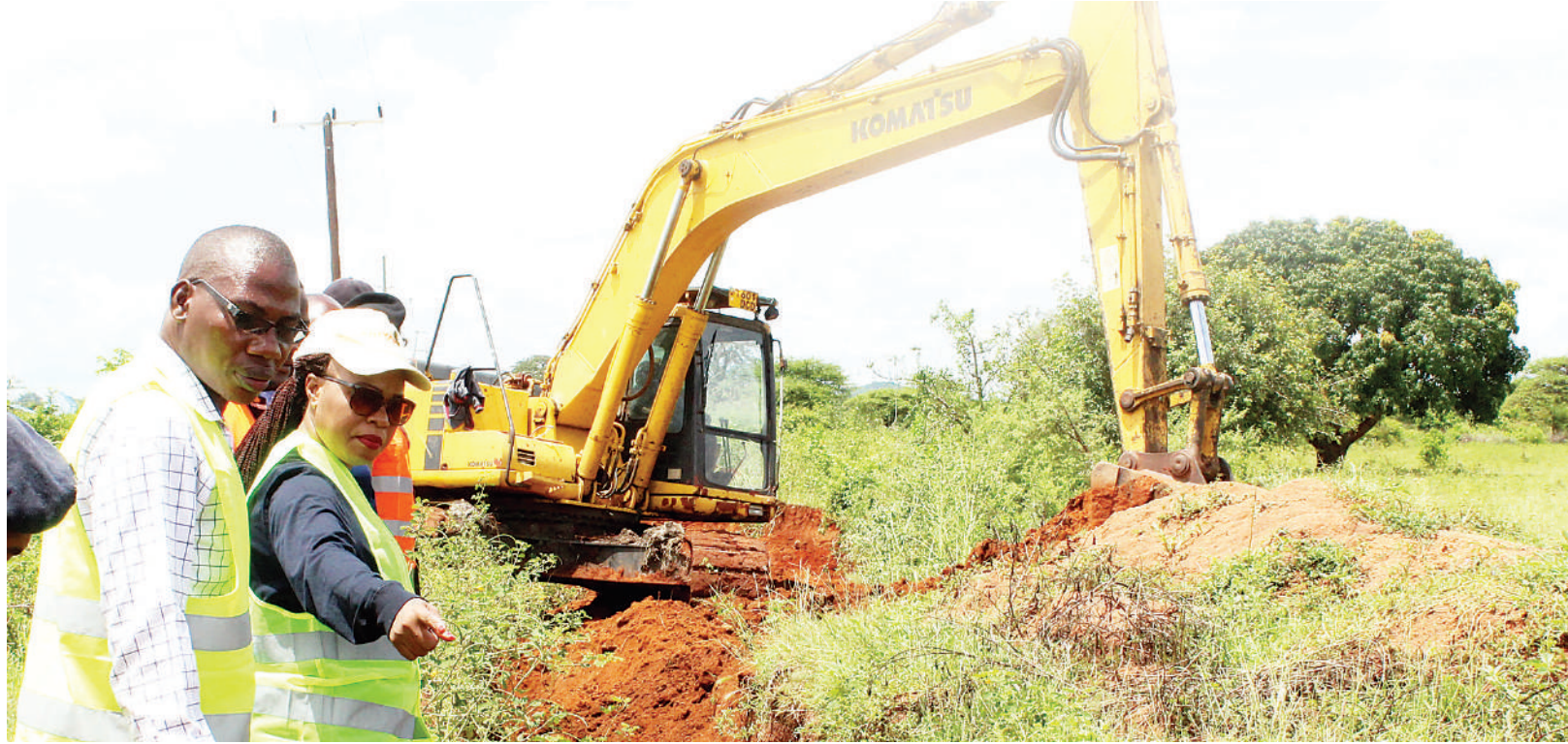
The laying of a Lake Victoria water project pipe is in progress, as witnessed in Masengwa ward, Shinyanga district, on Thursday. Photo: Correspondent Marco Maduhu
