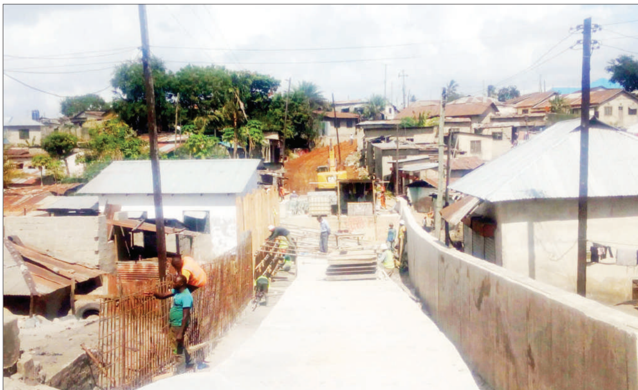
The construction of a bridge linking Keko Magurumbasi and Keko Mwanga wards in Dar es Salaam's Temeke municipality has made steady progress, as Correspondent Sabato Kasika confirmed at the weekend.
