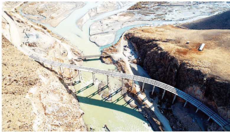
This aerial photo taken on Oct. 27, 2020 shows the construction site of the second phase of the north-south highway built by China in Kyrgyzstan.
