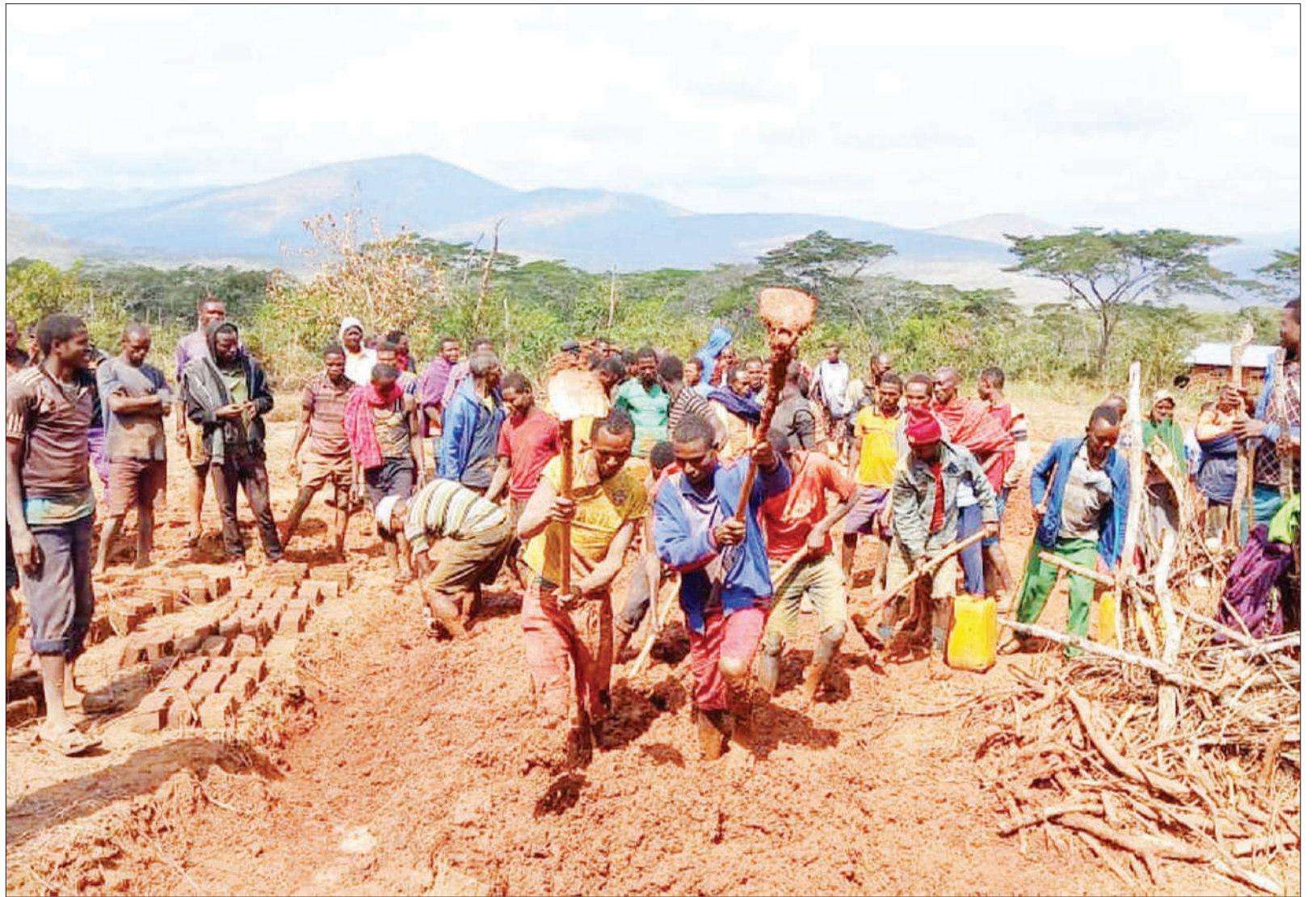
Residents of Ifuwa village in Kilolo District, Iringa Region, pictured yesterday making bricks for use in the construction of four classrooms at a local satellite school, whose completion will spare primary school pupils in the area the bother of having to walk some 20 km daily to and from the current Ifuwa Primary School. Photo: Correspondent Friday Simbaya
