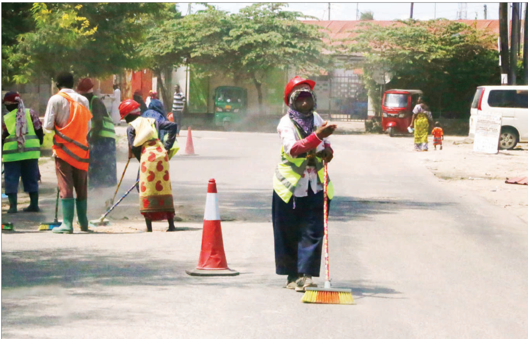
A member of road sweeper hire company directs traffic at Mwananyamala in Dar es salaam yesterday. Photo: Selemani Mpochi
