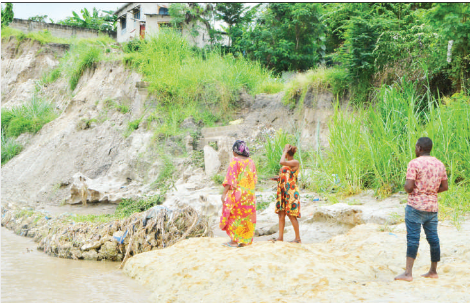
Residents of Goba on the outskirts Dar es Salaam witness evidence of the danger that the erosion the Mbezi River banks poses to houses in the neighbourhood. Photo: Correspondent Miraji Msala
