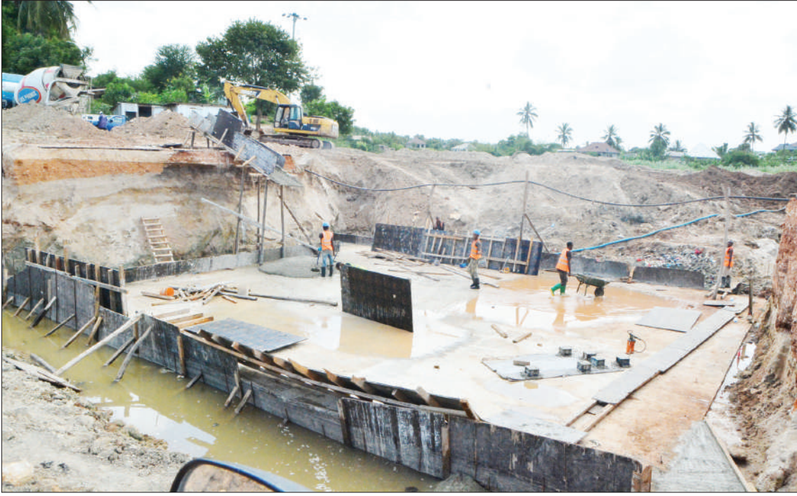
Expansion of Matosa bridge at Kimara in Ubungu District, Dar es Salaam, well under way – as found at the weekend. Photo: Correspondent Miraji Msala
