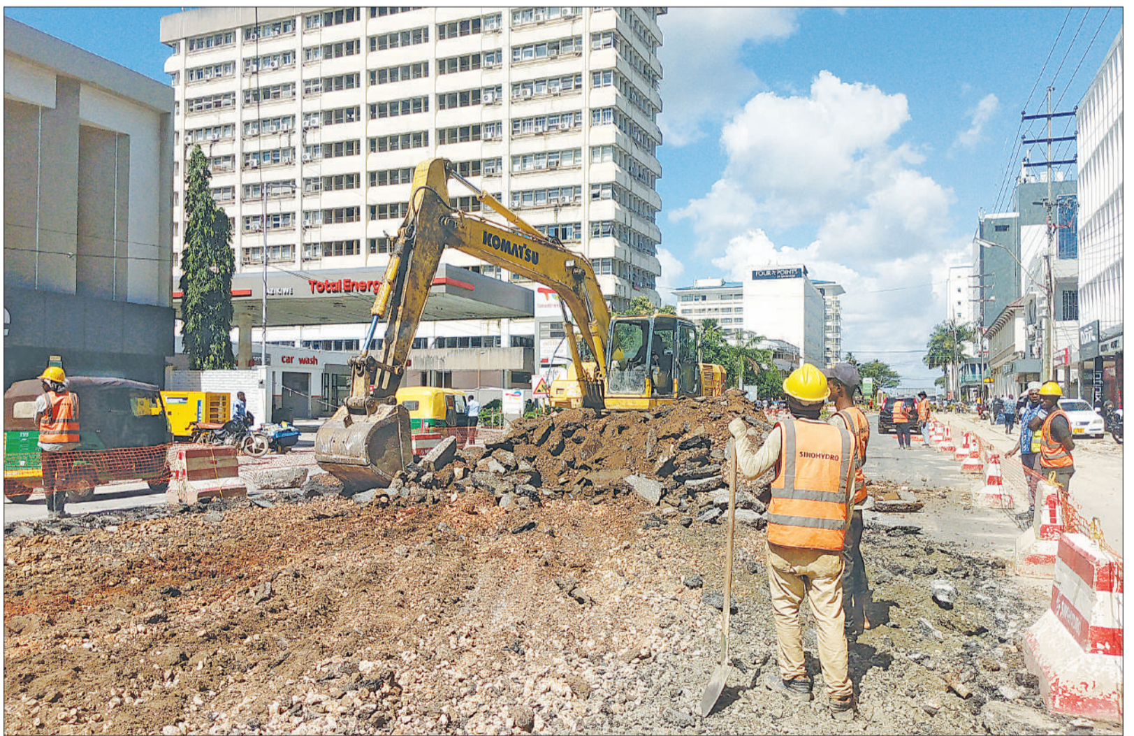
Expansion of Azikiwe Street in downtown Dar es Salaam well under way yesterday in implementation of the third phase of the city's rapid transit bus project. Photo: Correspondent Sabato Kasika
