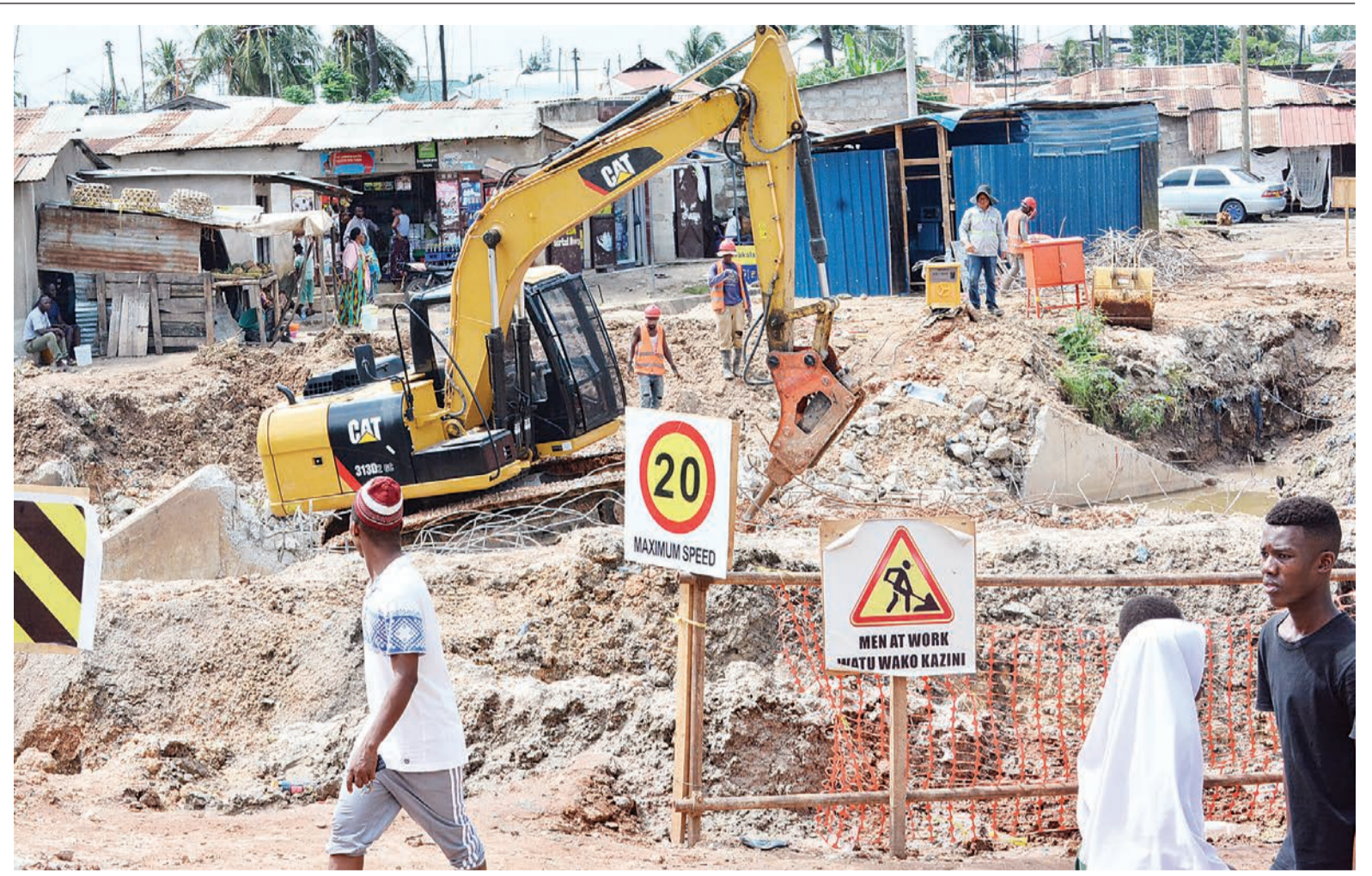
Construction of a bridge connecting Dar es Salaam's Kijitonyama and Manzese suburbs well in progress, as found on Tuesday. Photo: Correspondent Miraji Msala
