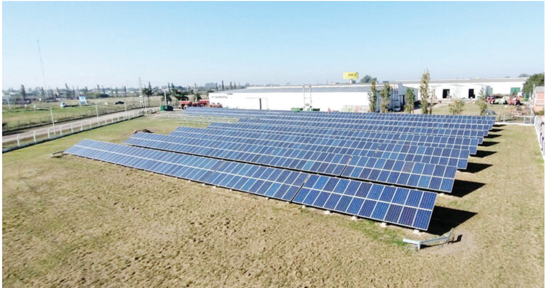
Photovoltaic panels in the solar park in the small town of Armstrong, in the Pampa region, the heart of Argentina's agricultural production. CREDIT: FARN
