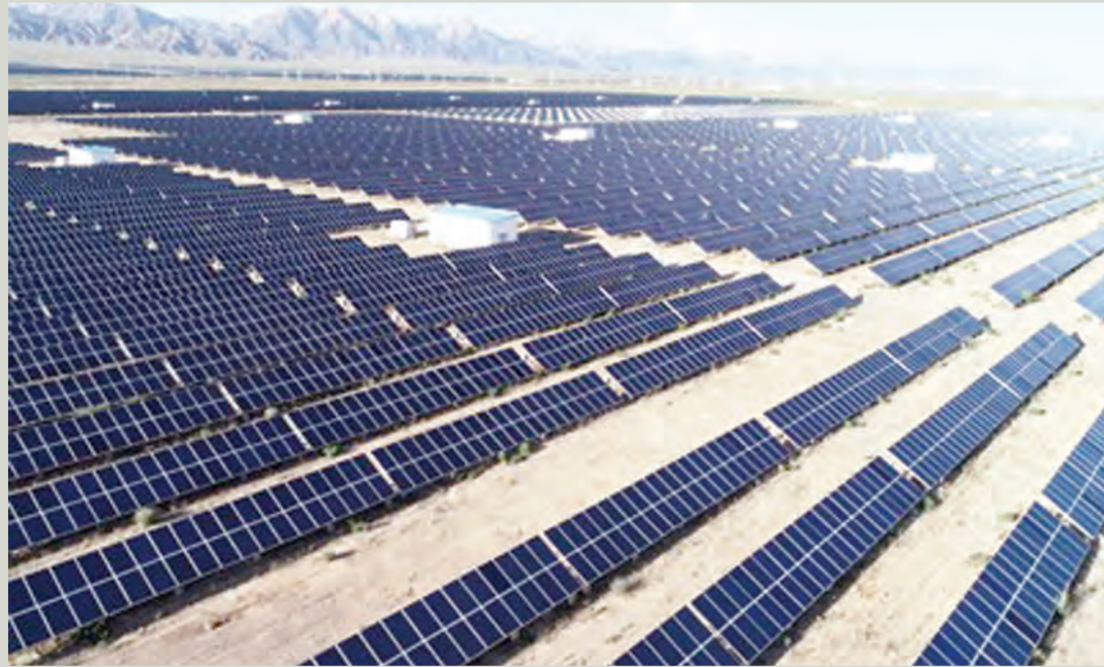
Photo taken on July 24, 2018 shows a photovoltaic (PV) power station in a photovoltaic industrial park in Delingha, Haixi Mongolian and Tibetan autonomous prefecture, northwest China's Qinghai province. (Photo by Wang Zheng/People's Daily Online)
