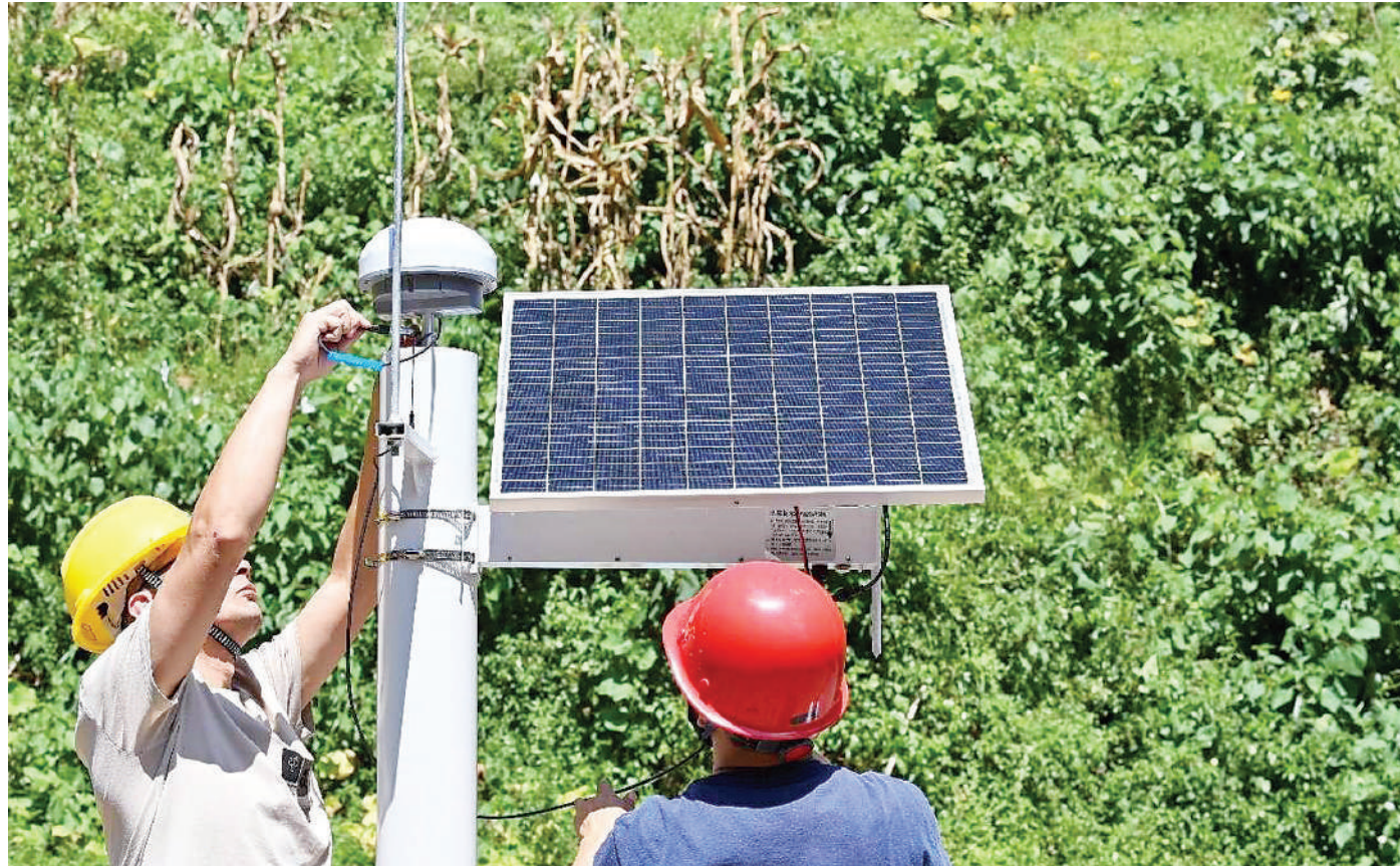
A geological monitoring device enabled by the BeiDou Navigation Satellite System is installed in Nanmu township, Youyang Tujia and Miao autonomous county, southwest China's Chongqing municipality. (People's Daily Online/Qiu Hongbin)
