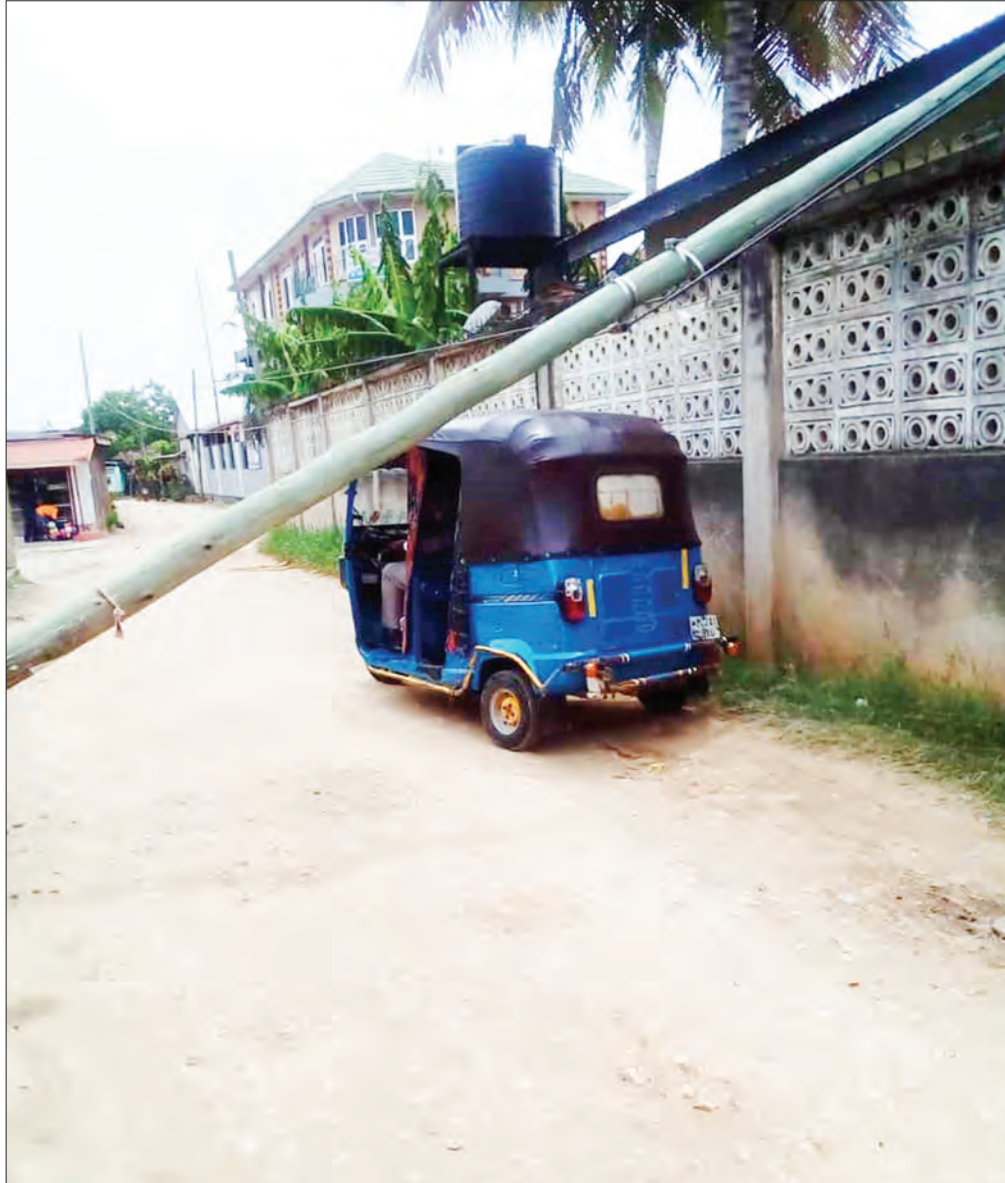
This post, which is supposed to support telephone lines, is installed near the primary court in Dar es Salaam's Manzese-Sinza suburb. It just could not withstand the ferocity of the strong winds experienced in parts of the city last week and has been lying in this state since, closing the particular section of the road to vehicular traffic. Photo: Guardian Correspondent
