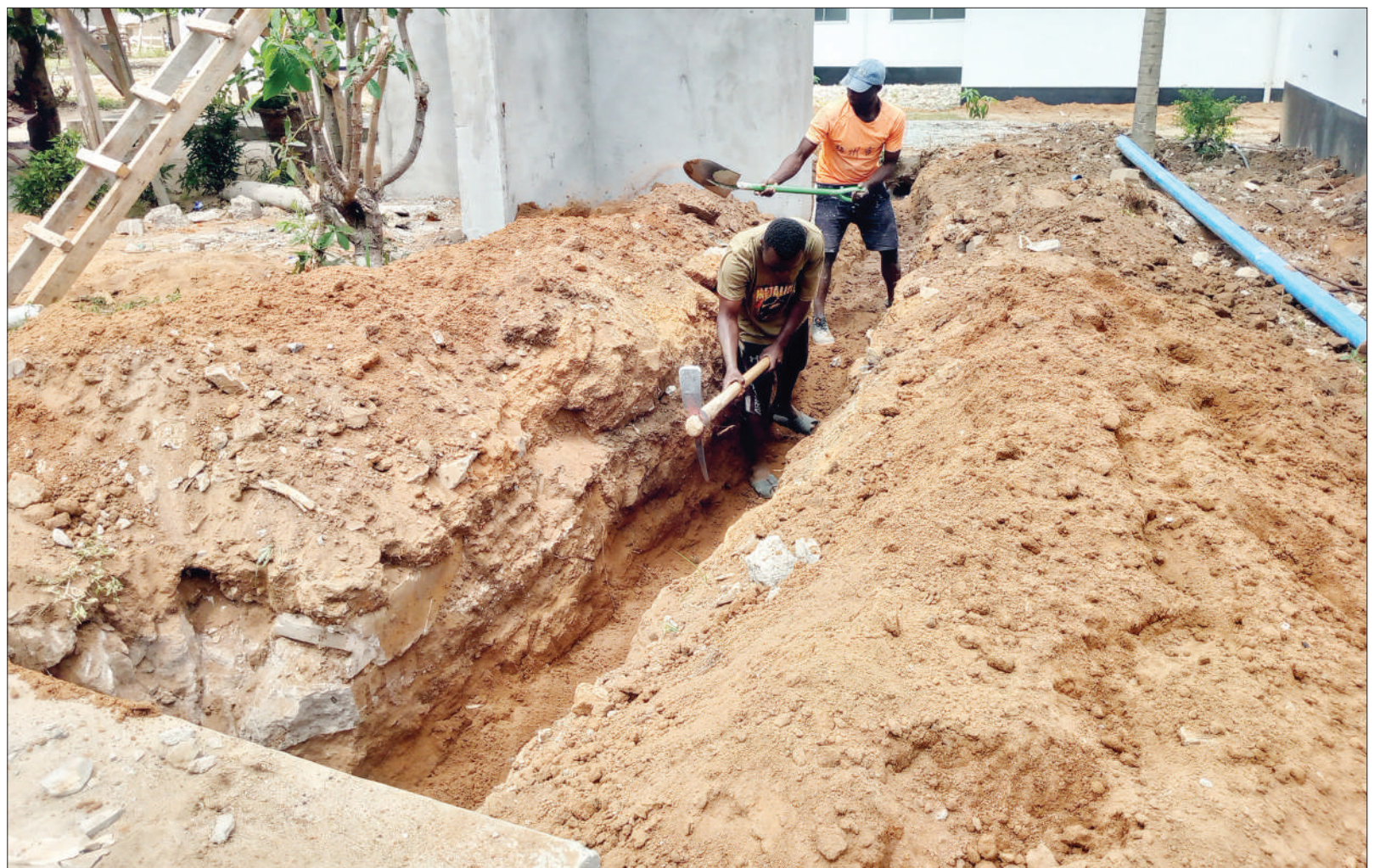
The digging of a trench to pave the way for the installation of sewage pipes to serve a health centre in Dar es Salaam's Majohe ward gets under way earlier this week. The centre is expected to start work next month. Photo: Correspondent Sabato Kasika
