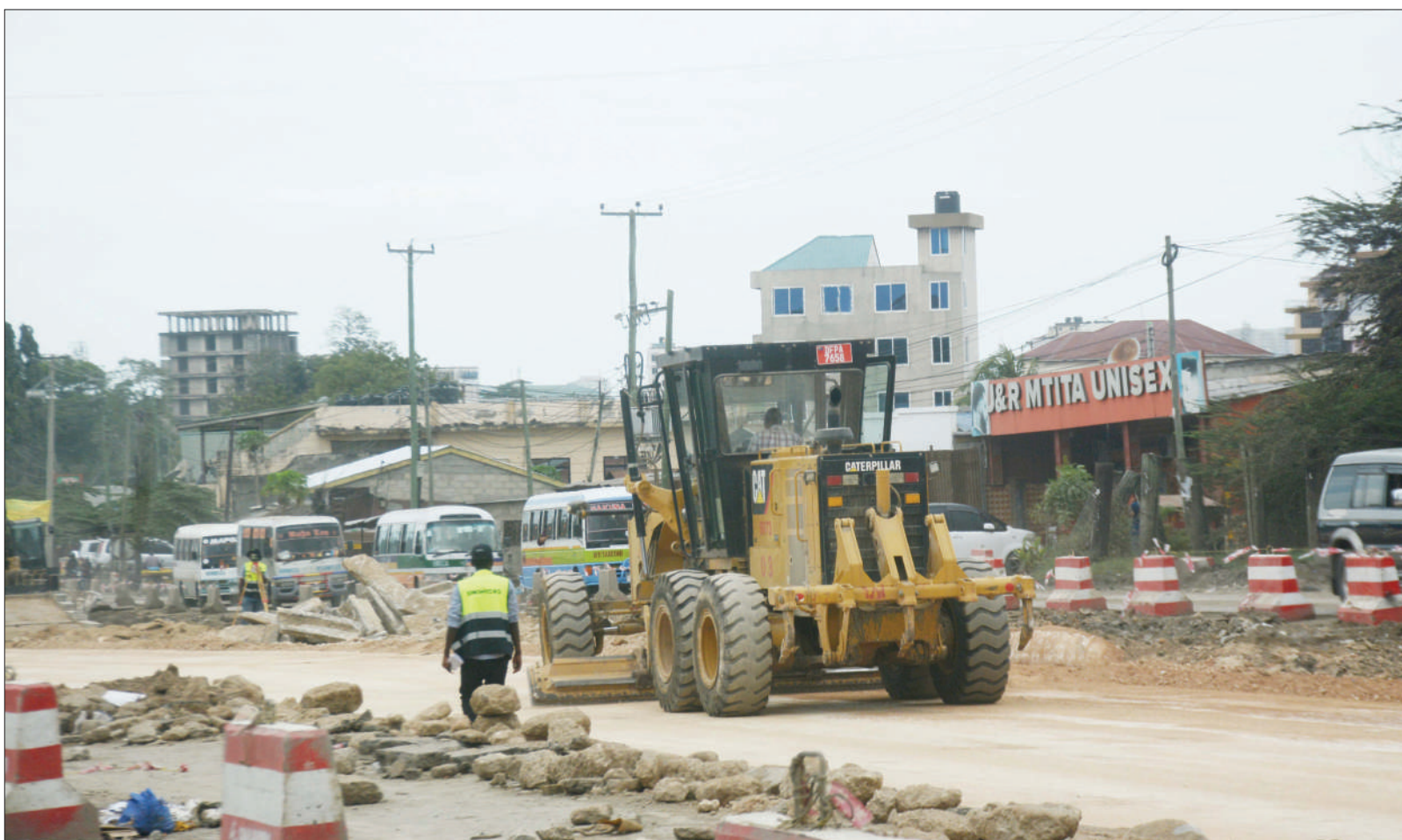
A grader deployed by Sinohydro Company contractors at work at an Ilala section of Dar es Salaam's Uhuru Road earlier this week as preparations for the construction of Bus Rapid Transit project infrastructure continued. Photo: Correspondent Jumanne Juma
