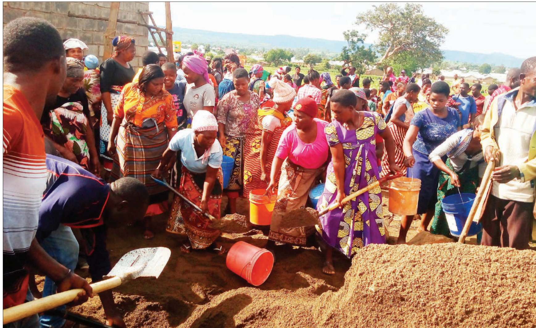
Utengule - Usongwe ward residents in Mbeya region join volunteer to collect sand for the construction of nine classrooms at Usongwe secondary school aiming at accommodating 400 students selected to join Form One this year. Photo: Correspondent Nebart Msokwa
