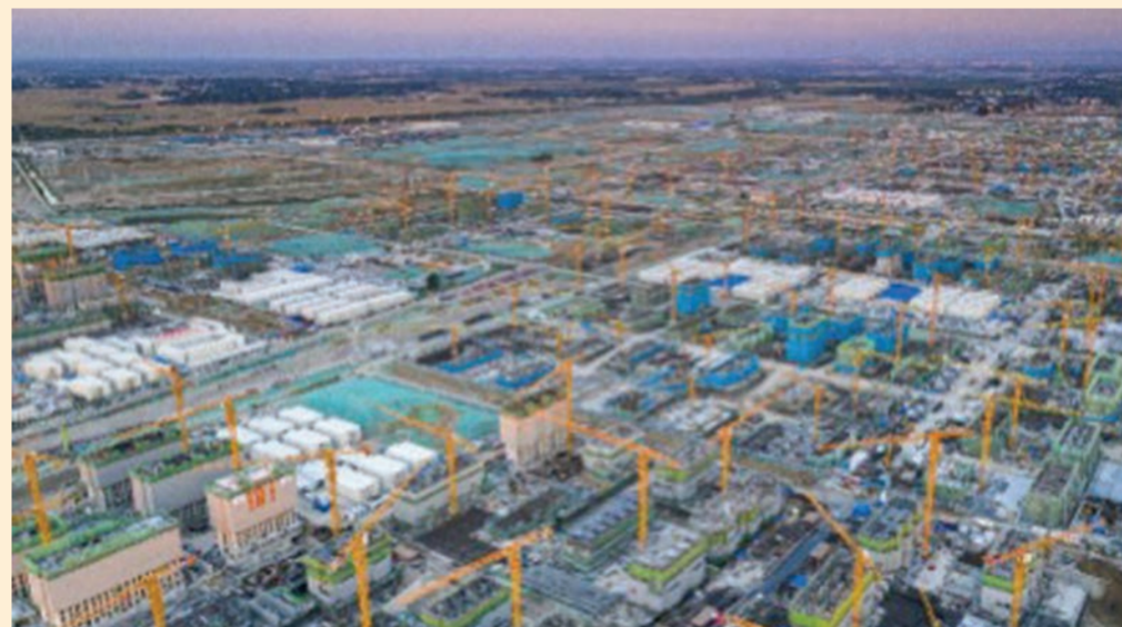
Construction of the Rongxi Zone of Xiong'an New Area, north China's Hebei province, is in full swing, June 20, 2021. File photo
