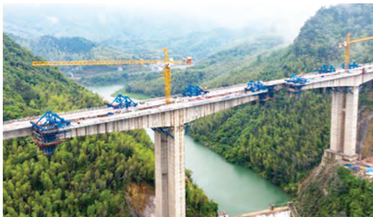
A super large bridge along the Pingxiang-Lianhua expressway in Pingxiang, east China's Jiangxi province is being constructed, May 4, 2021. (File photo)
