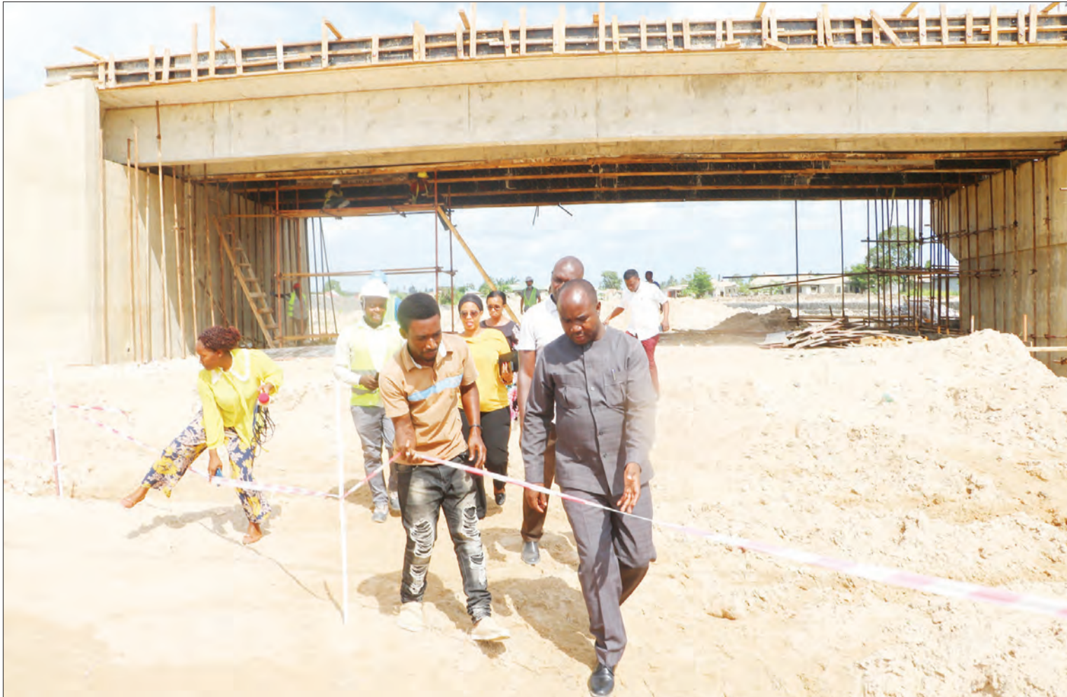
Ijala district commissioner Ng'wilabuzu Ludigija (R) pictured at the weekend at the site of suburban Dar es Salaam's Ulongoni B bridge, which is being built by Chinese firm Chongkwi International. Photo: Correspondent Jumanne Juma
