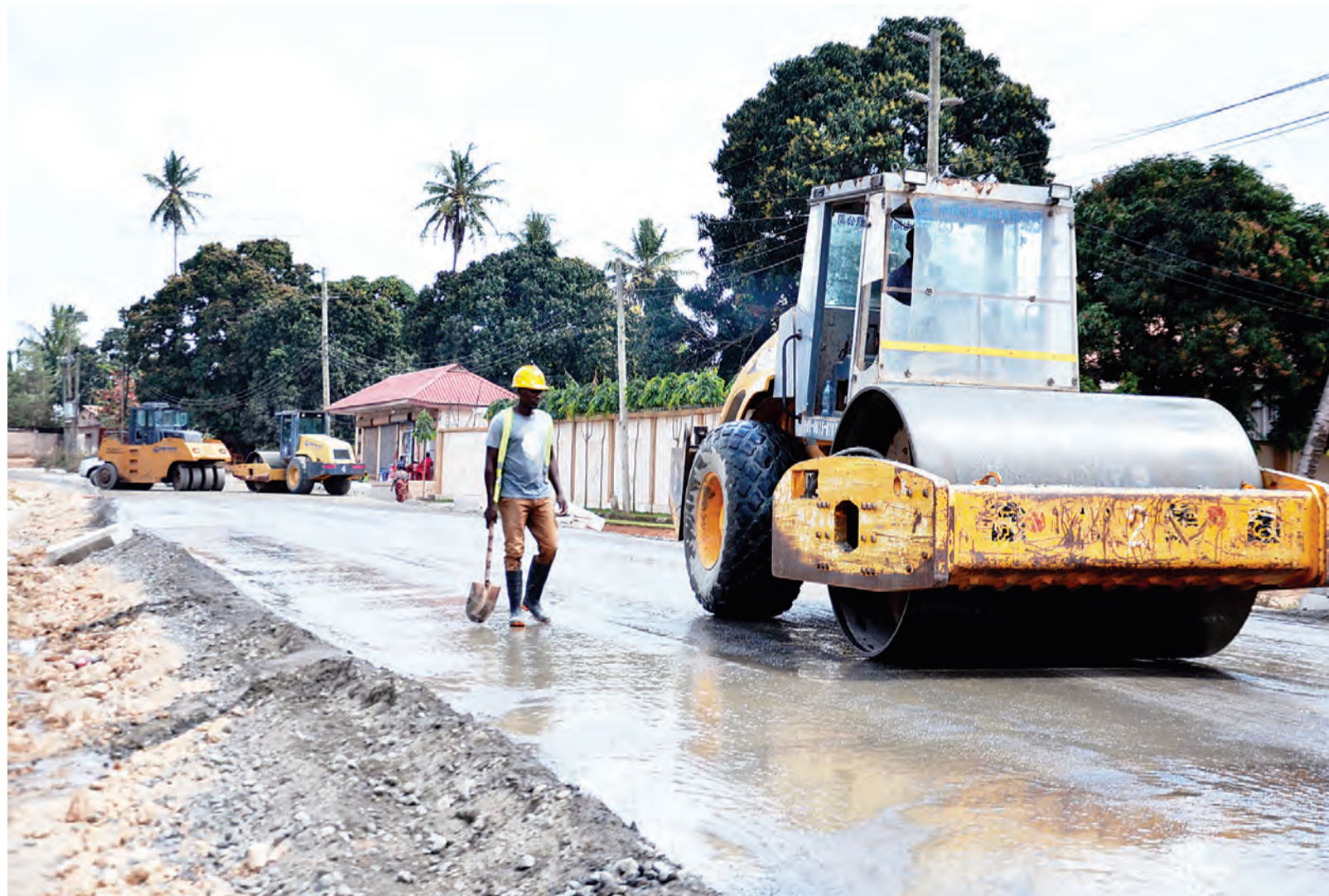
Construction of a road to tarmac level well under way in Dar es Salaam's Kinyerezi suburb earlier this week. Photo: Correspondent Jumanne Juma
