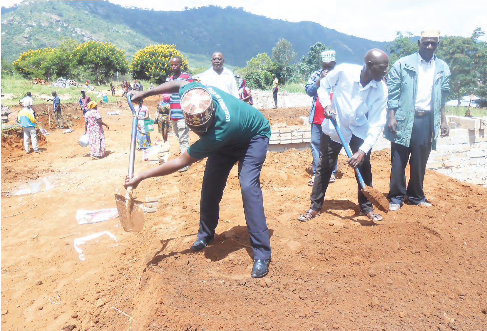
Residents of Songe ward in Kilindi District, Tanga Region, pictured earlier this week taking part in preparing the groundwork for the construction of a building to accommodate classes for Forms Five and Six students at Seuta Secondary School. Photo: Correspondent Dege Masoli
