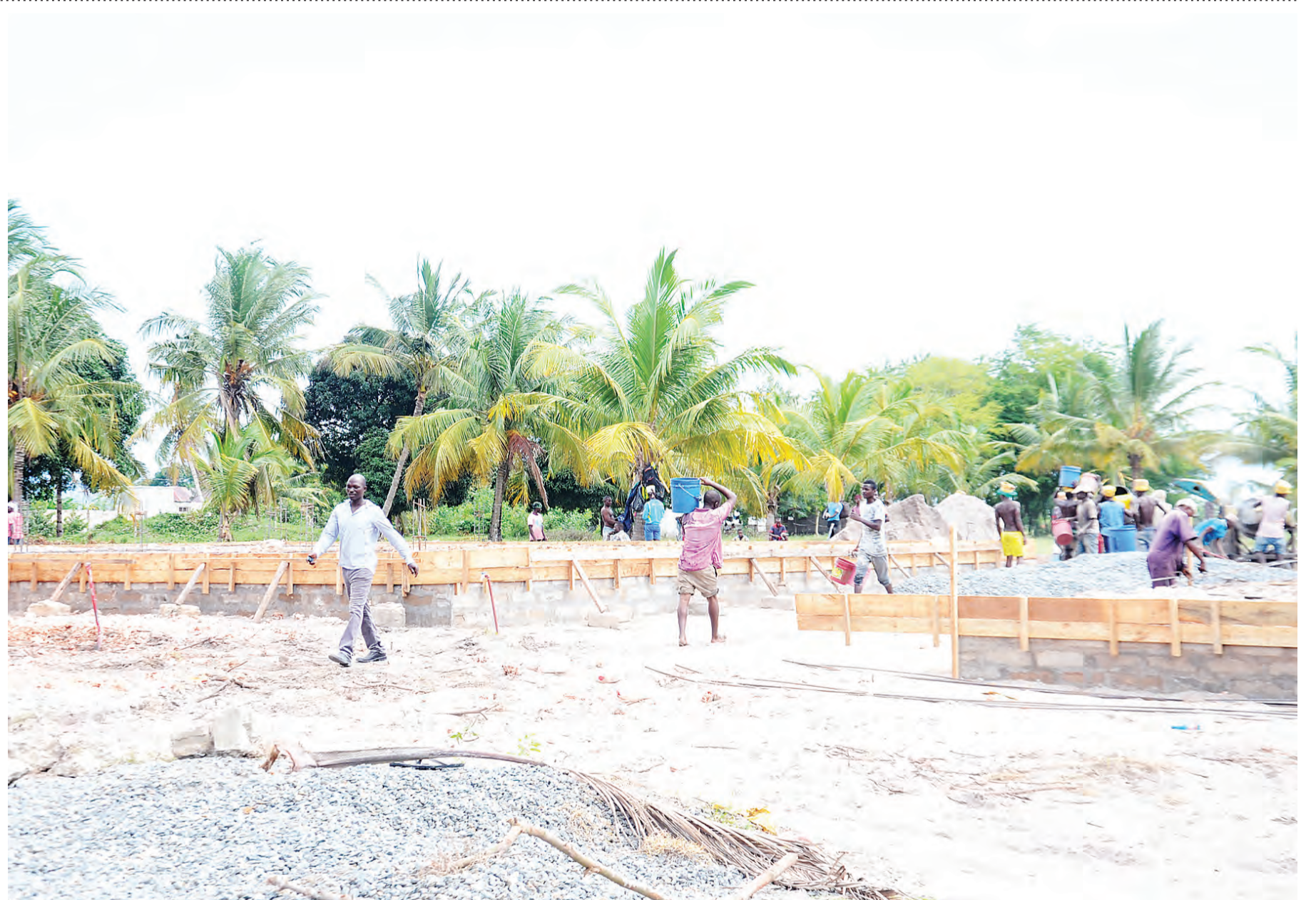
Construction of a hospital at Kivule in Ilala District, Dar es Salaam Region, gets under way. Correspondent Jumanne Juma captured the scene earlier this week.
