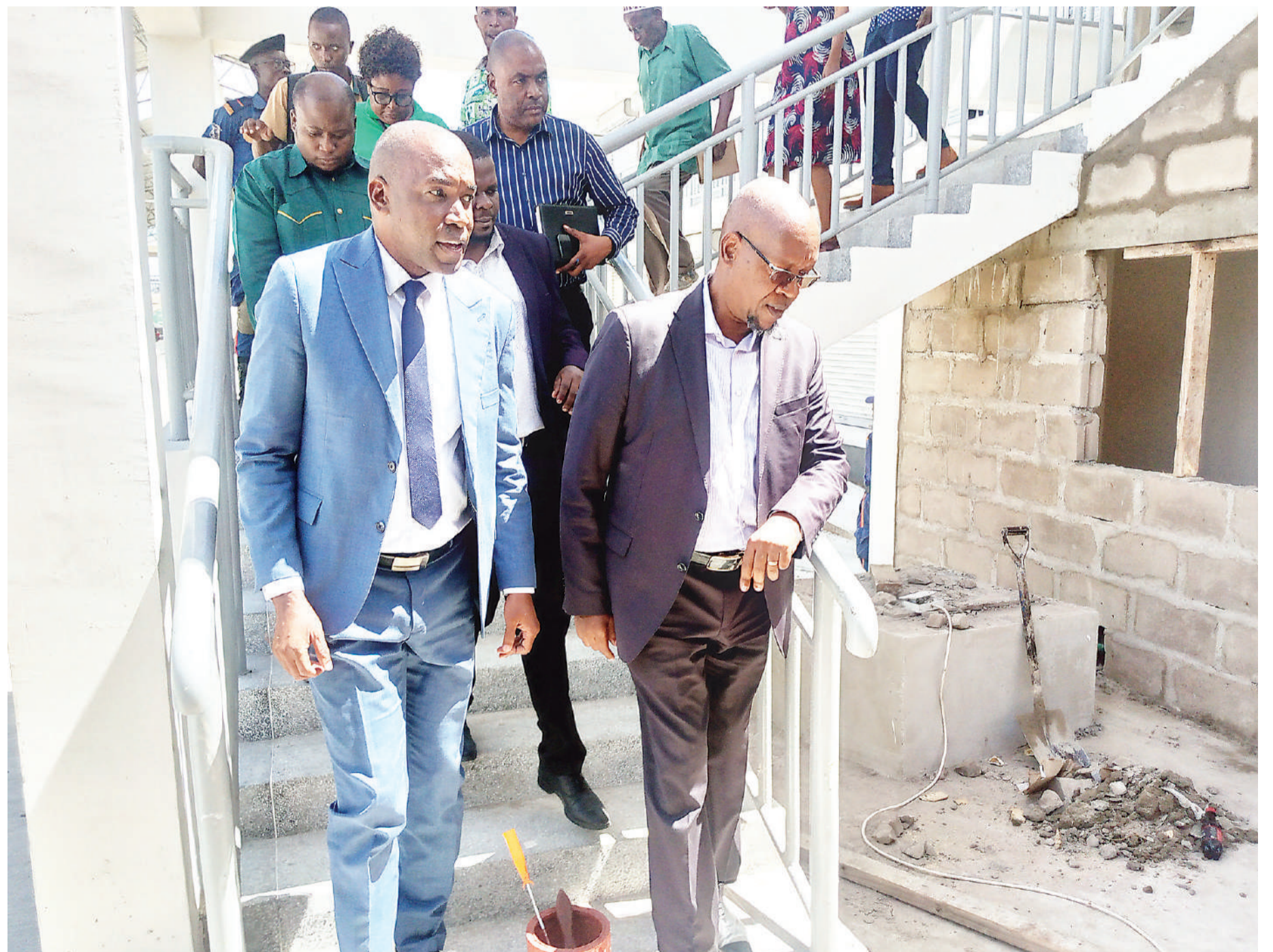
Temeke district commissioner Mobhare Matinyi (R) and other leaders on an assessment tour of progress in the ongoing construction of Dar es Salaam's Mbagala Zakhem market yesterday. Photo: Correspondent Sabato Kasika
