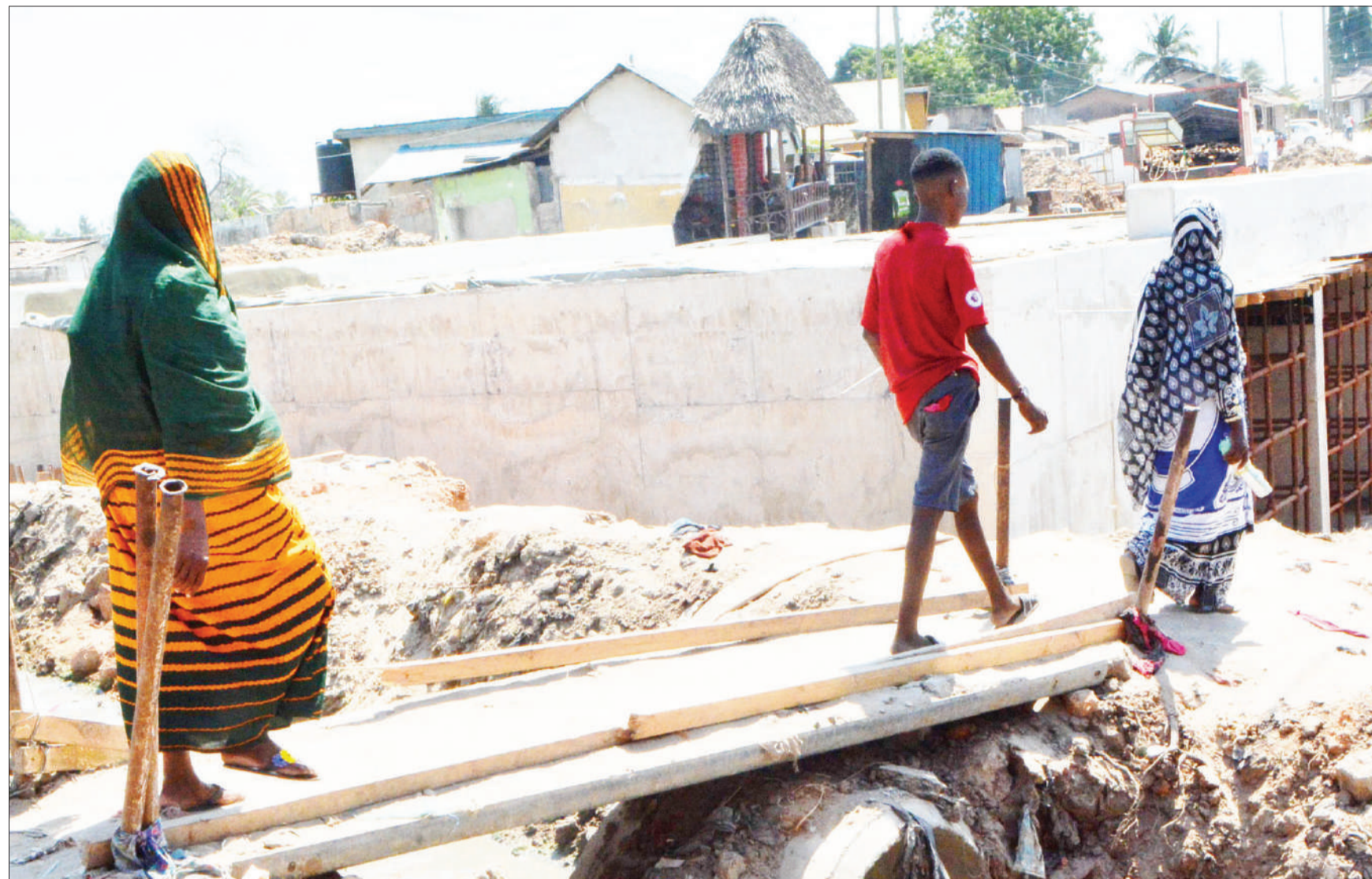
Residents of Tandale and Kijitonyama in Dar es Salaam make do with a makeshift bridge connecting the two suburbs to Kwa Ali Maua yesterday owing to ongoing construction of a permanent one. Photo: Correspondent Miraji Msala
