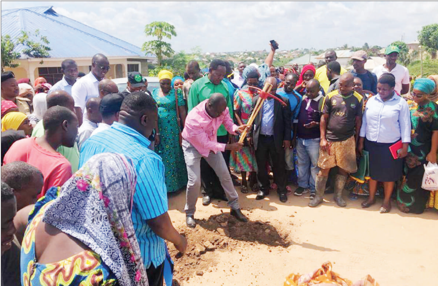
Water minister Jumaa Aweso participates in digging a water pipe channel at Golani Kimara Ward in Ubungo District which is under Dar es Salaam Water and Sanitation Authority. Photo: Guardian Correspondent
