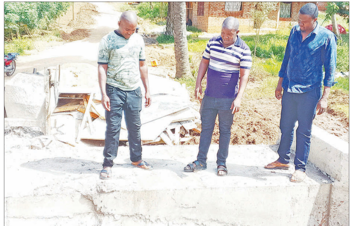
Mukadam Sabuni (C), Councillor for Majengo Ward in Muheza District, Tanga Region, in discussion with Tanzania Rural and Urban Roads Agency engineer Judica Athanas (R) during a visit to inspect construction of a culvert at Mdote Street yesterday. Photo: Correspondent Steven William
