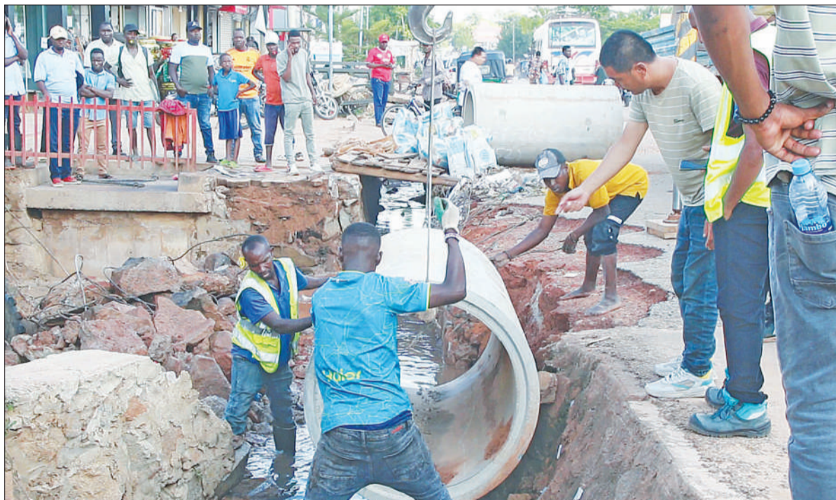
Contractor of a project under the Tanzania Cities Infrastructure Improvement Project (TACTIC) in Kahama Municipal Council, Shinyanga Region, puts culvert at the drainage channels to prevent water from entering residential areas at Nyasubi Street yesterday. Photo: Correspondent Shaban Njia
