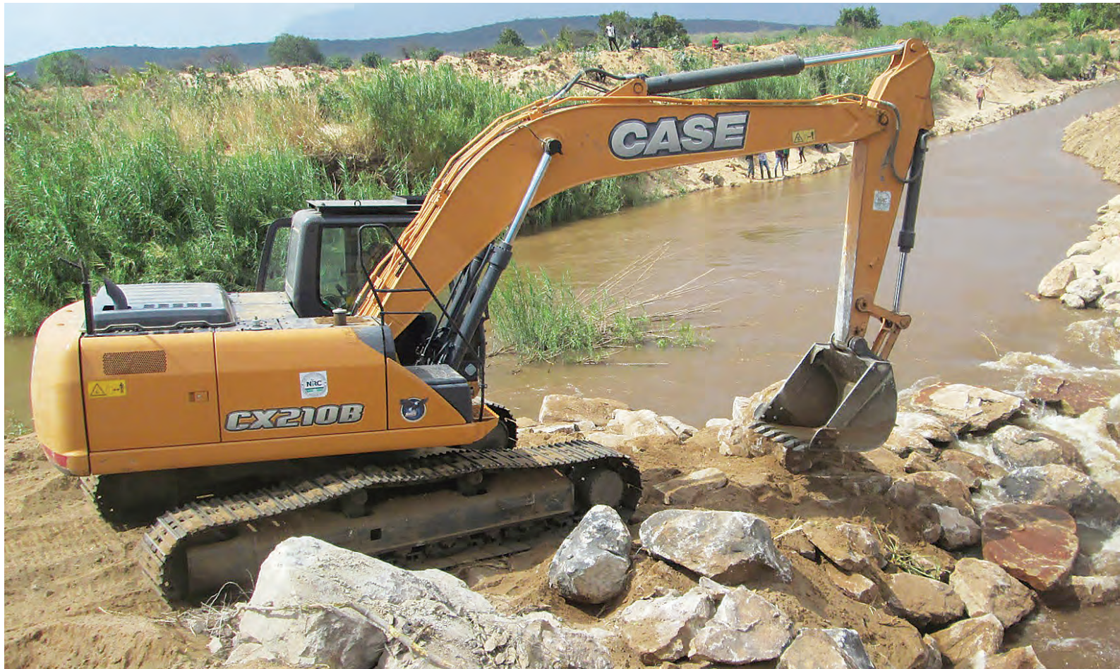
An excavator is deployed in efforts to direct Lukosi River in Kilolo District, Iringa Region, back to its normal course – as found earlier this week. The river feeds into the Great Ruaha River, which plays a crucial role in irrigation farming. The diversion was caused by last season's floods. Photo: Correspondent Oscar Asenga
